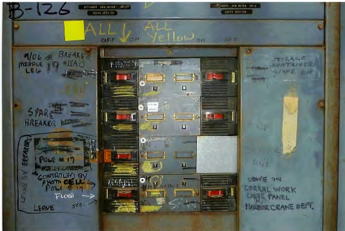
Electrical Panel B-126
