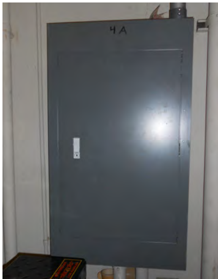
Example of electrical panel at POLA with no shock hazard ID labels on it.
