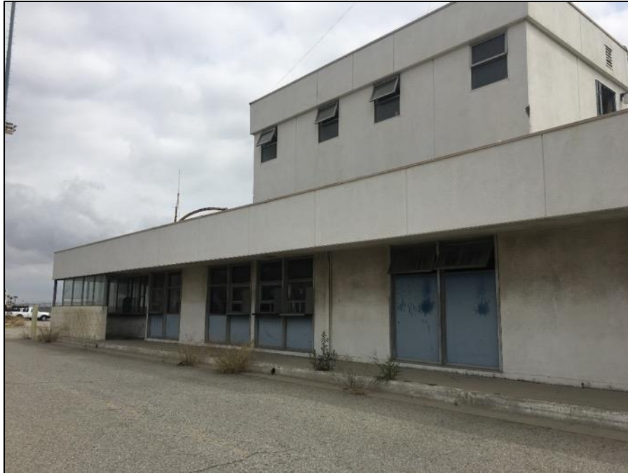
Figure 7. North end of the west façade of the Gate Office Building, view north (SWCA, 2018).
