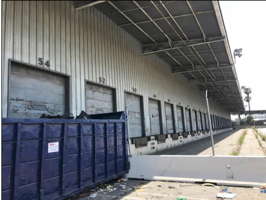
Figure 22. East portion of the south façade of the Consolidated Freight Station, view northeast (SWCA, 2018).
