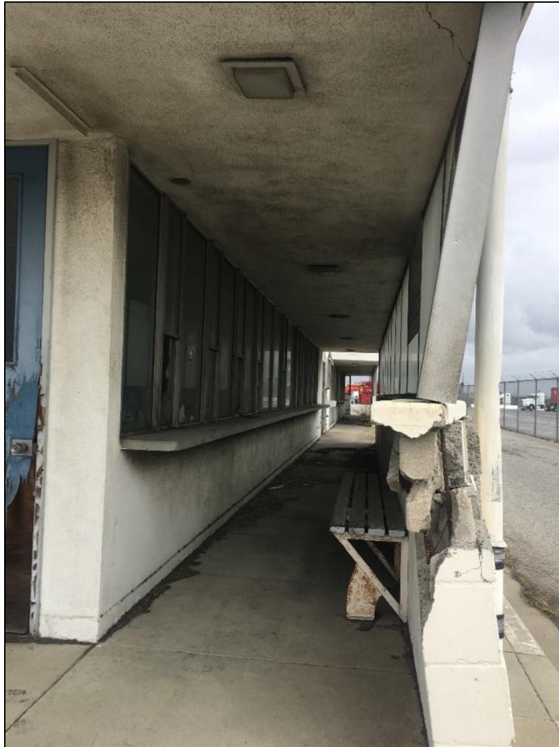
Figure 11. Detail of enclosed walkway on east façade of the Gate Office Building, view north (SWCA, 2018).
