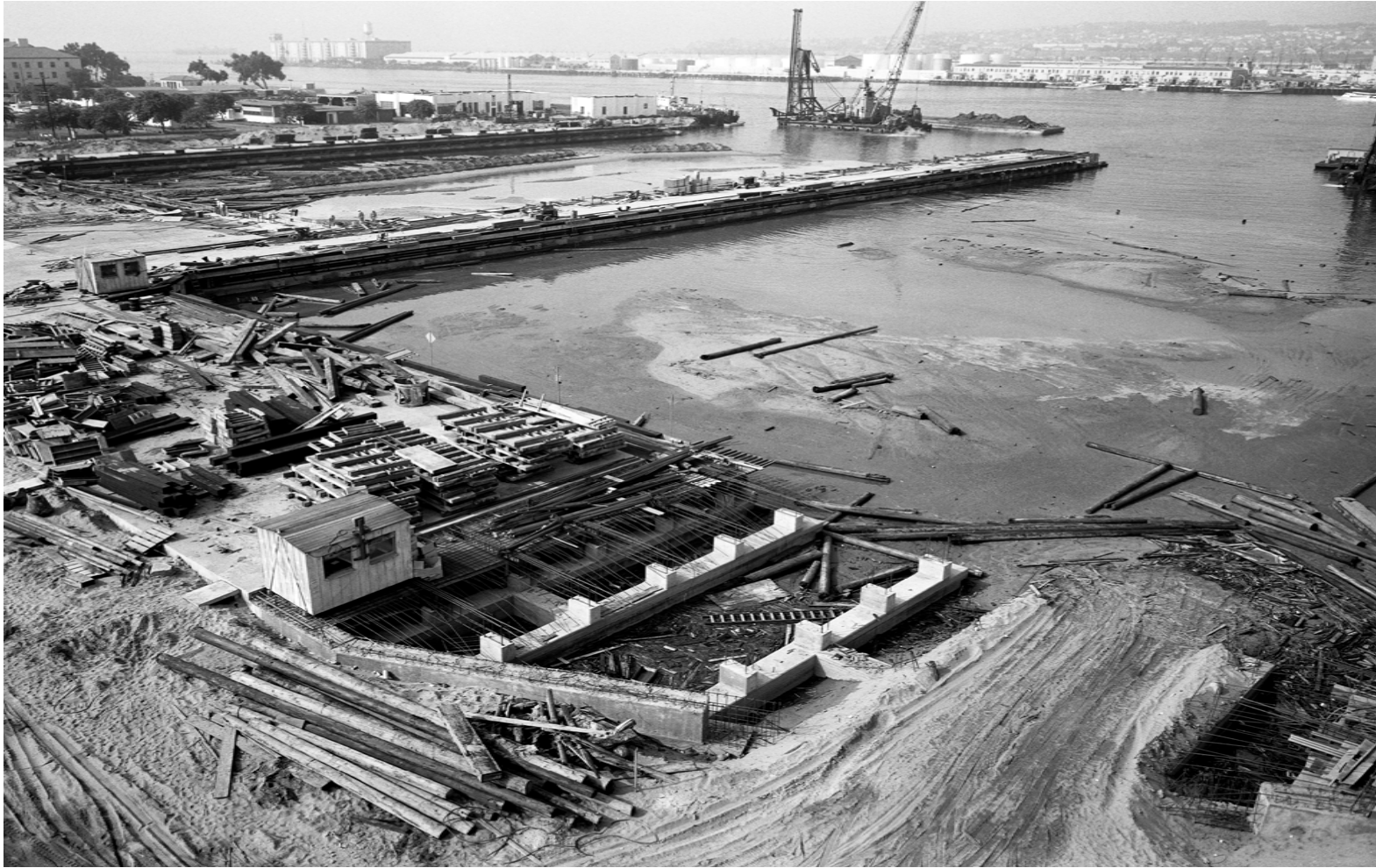
Figure 3 - This photo from 8/18/1960, looking southwest, shows extensive modifications by Bethlehem Steel. The World War II-era slipways were converted into basins in 1959–1961 as Bethlehem Steel transformed its former wartime shipbuilding operation into a ship repair and conversion facility. The slipways and two of the Colby cranes constructed during World War II were removed.
