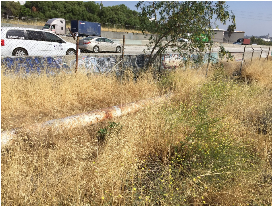
Photo 38 – Pipeline and adjoining freeway. Aboveground tanks from the adjoining tank far visible in the background.
