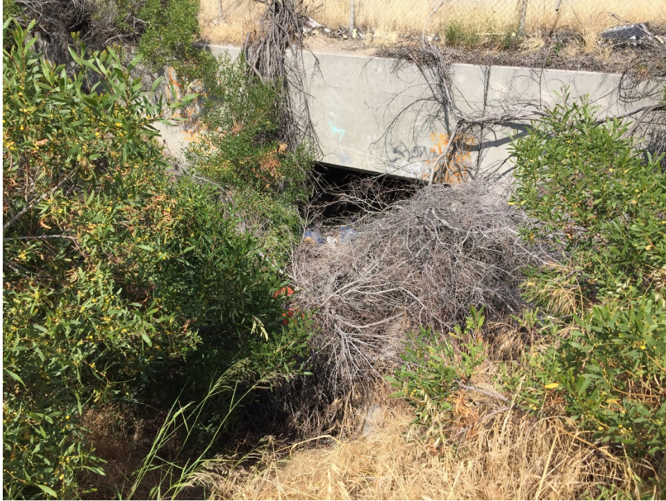
Photo 31 – A concrete culvert opening on the northwestern edge of the Property. Stormwater flows onto the Property from beneath the freeway.
