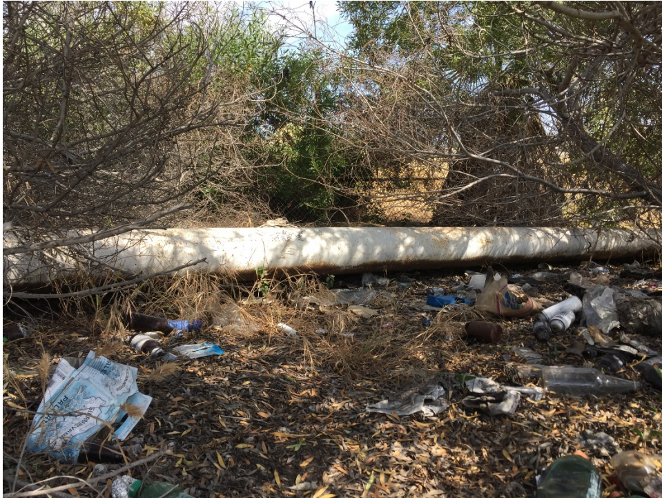
Photo 24 – Pipelines and trash from past homeless encampment activity on the Property.
