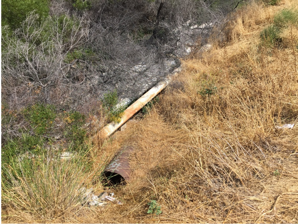
Photo 29 – Pipelines and corrugated metal piping.
