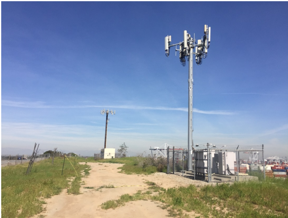
Photo 6 – Cellular towers and associated electrical equipment located on the central portion of the Property.
