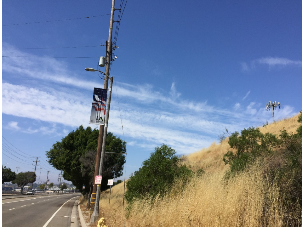
Photo 53 – One pole-mounted transformer is located along the southeastern edge of the Property.
