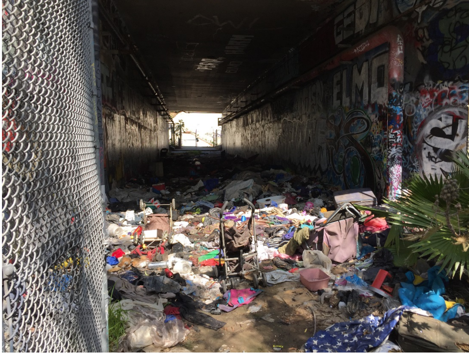
Photo 43 – Culvert beneath the freeway filled with trash and evidence of a homeless encampment.
