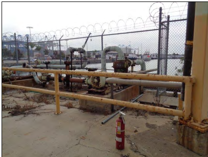
Figure 20: Star-Kist Plant No. 4, ancillary/related buildings/structures adjacent to south elevation, showing pipes, railings, fencing, and concrete pads, camera facing southeast. ICF, 2018.
