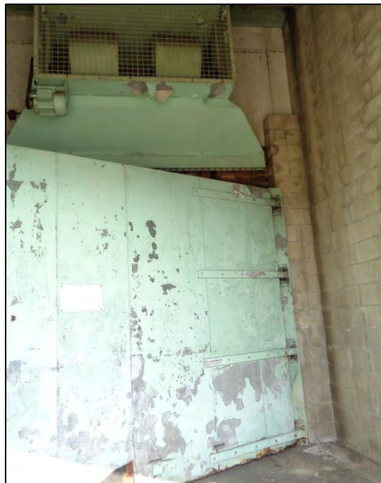
Photograph 6: South elevation, Cold Storage portion of the facility, detail showing a cold storage door, camera facing northeast. ICF, 2018.
