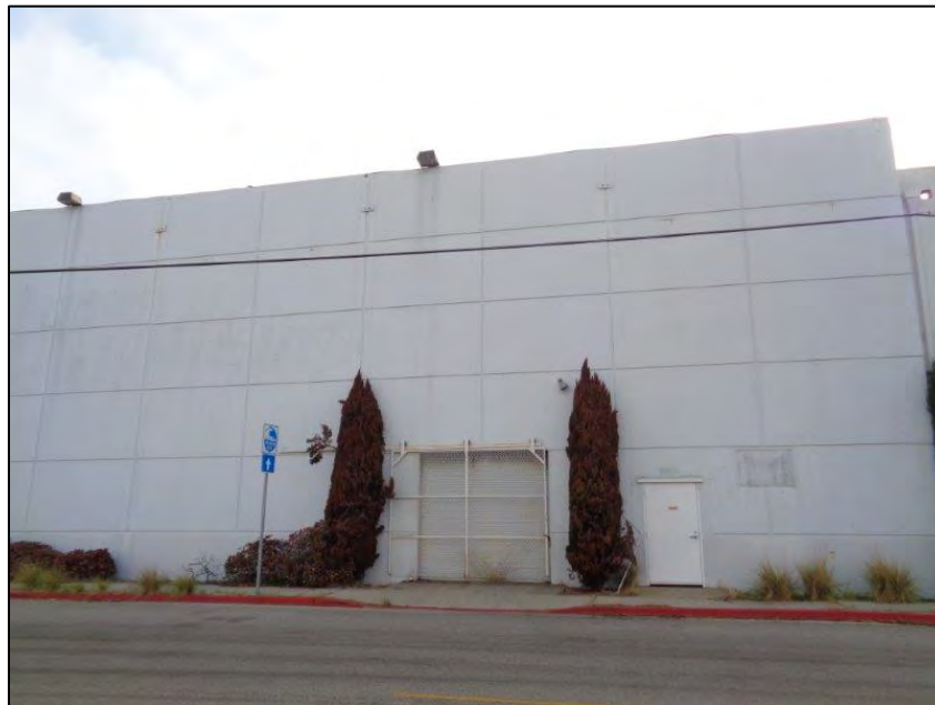
Figure 8: Star-Kist Plant No. 4, primary (west) elevation, detail of second volume from the north, camera facing east. ICF, 2018.
