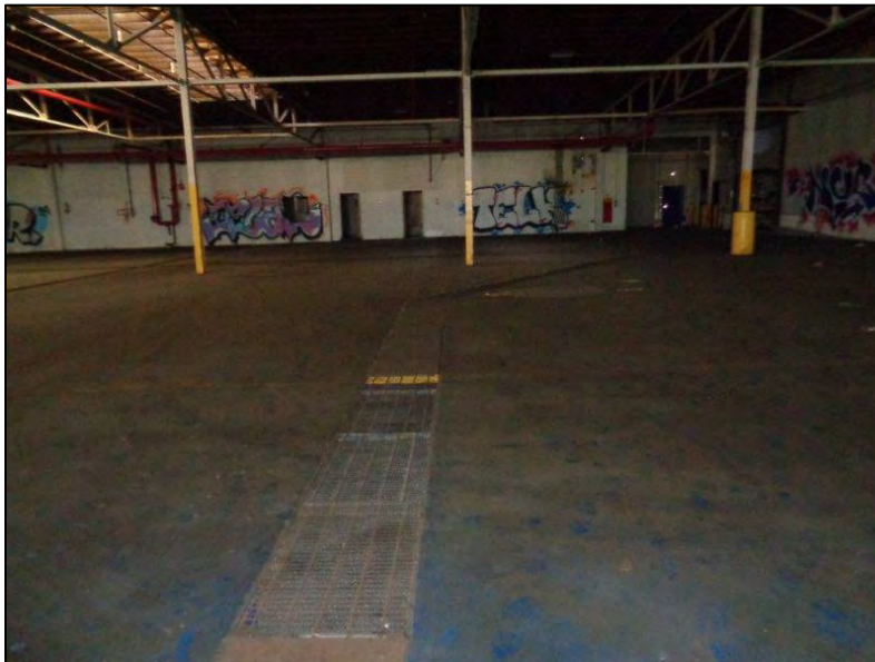
Figure 28: Star-Kist Plant No. 4, interior, warehouse/manufacturing area showing drains in floor, camera facing east. ICF, 2018.
