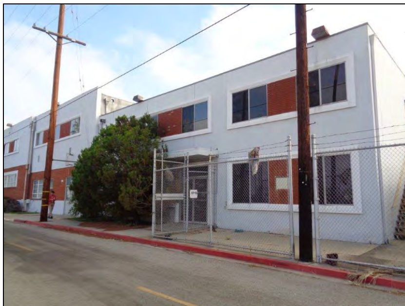
Figure 5-11. Star-Kist Plant No. 4, primary (west) elevation, detail of fifth volume from the north, camera facing northeast.
