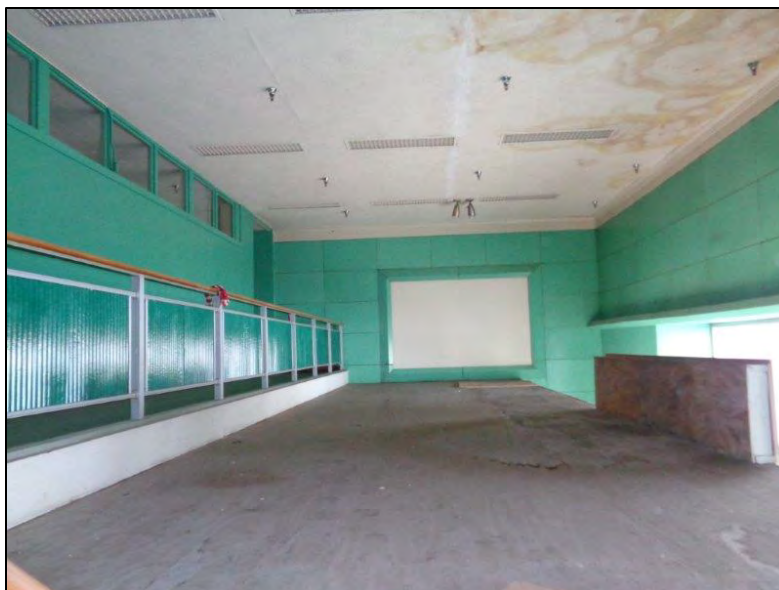
Figure 5-27. Star-Kist Plant No. 4, interior, entrance lobby shown from staircase landing, camera facing south. ICF, 2018.
