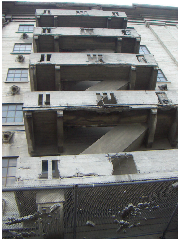
Figure 7 – Exterior Stair Deterioration
