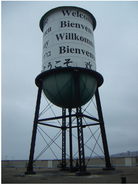
Figure 16 – Water Tank on Roof
