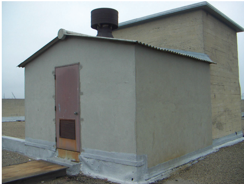
Figure 19 – Equipment Building on Roof
