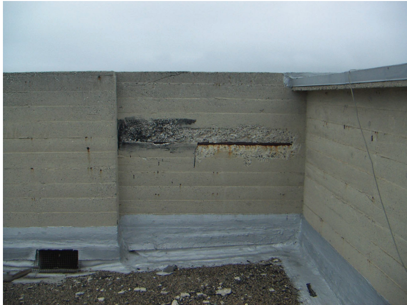
Figure 8 – Roof Parapet Deterioration
