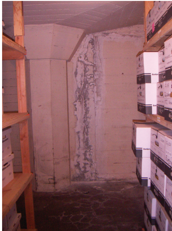
Figure 3 – Water Damage at Exterior Wall on Second Floor
