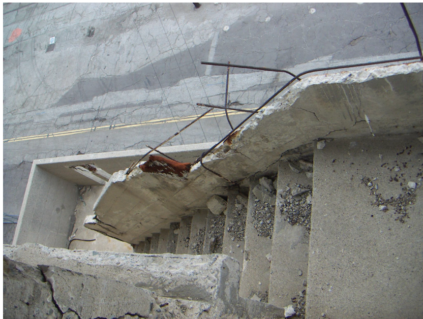
Figure 5 – Exterior Stair Deterioration
