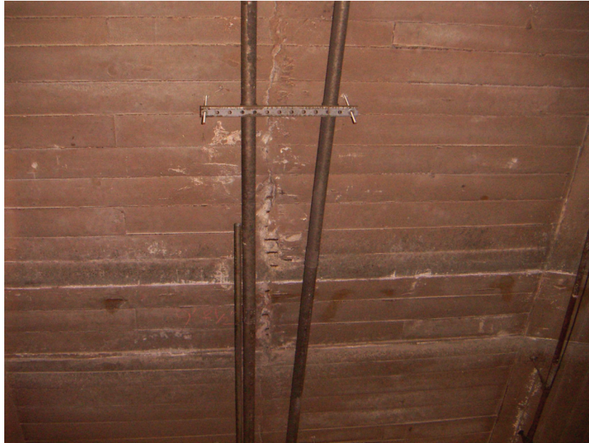
Figure 2 – Floor Crack at Ceiling of First Floor
