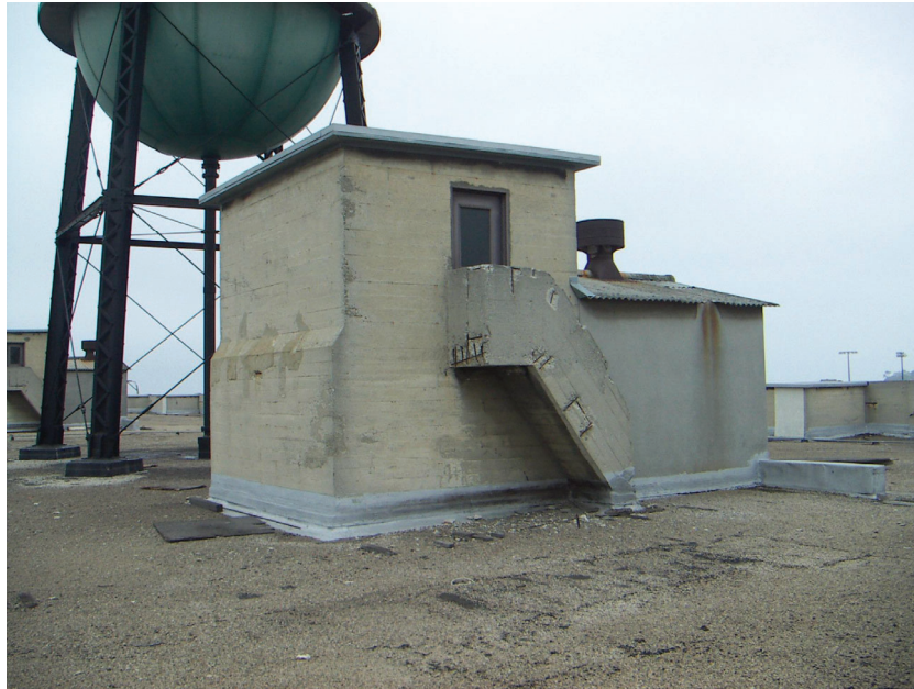
Figure 18 – Equipment Building on Roof
