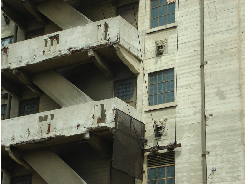
Figure 4 – Exterior Stair Deterioration
