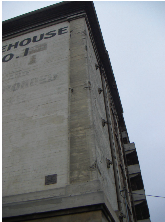
Figure 9 – Northwest Corner Deterioration & Historical Plaque
