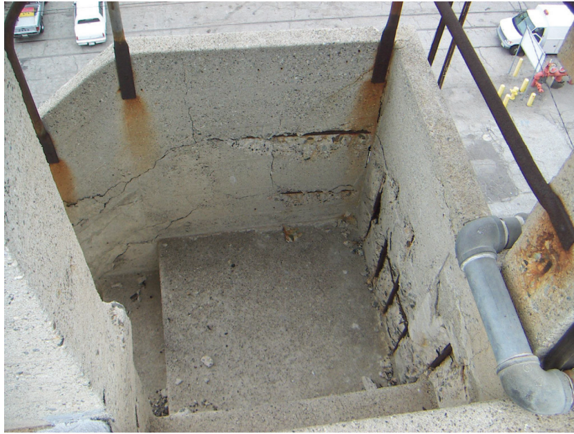
Figure 6 – Exterior Stair Deterioration
