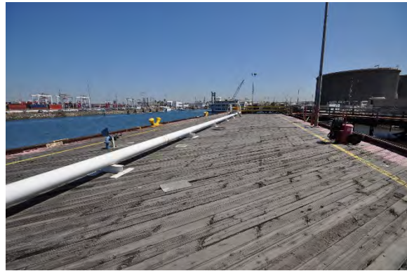
Figure 6: View looking north at timber wharf along Berth 163; Tank Farm 1 at right. (GPA, 2018)
