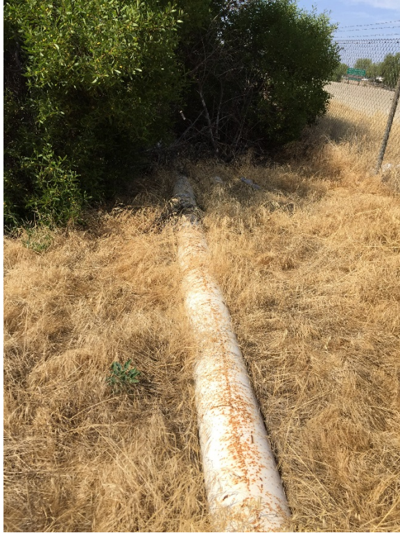
Photo 35 – Only one pipeline was visible on the northern portion of the Property.
