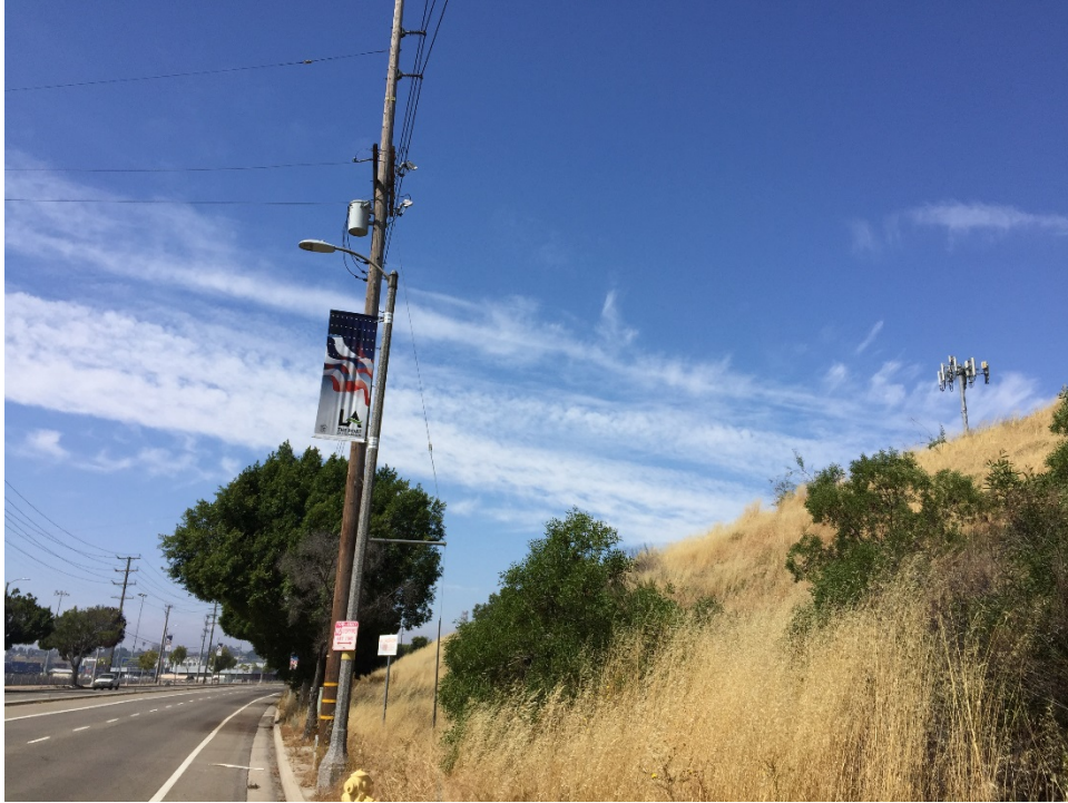
Photo 53 – One pole-mounted transformer is located along the southeastern edge of the Property.
