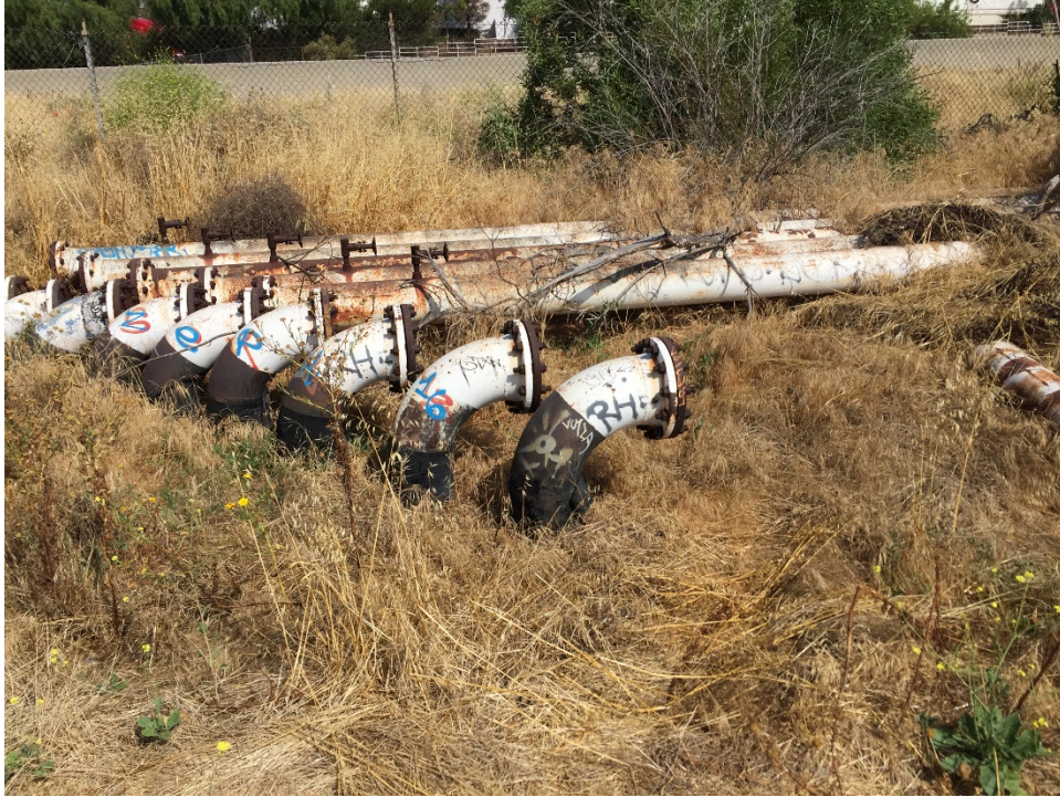
Photo 23 – Pipeline infrastructure on the central-western portion of the Property.
