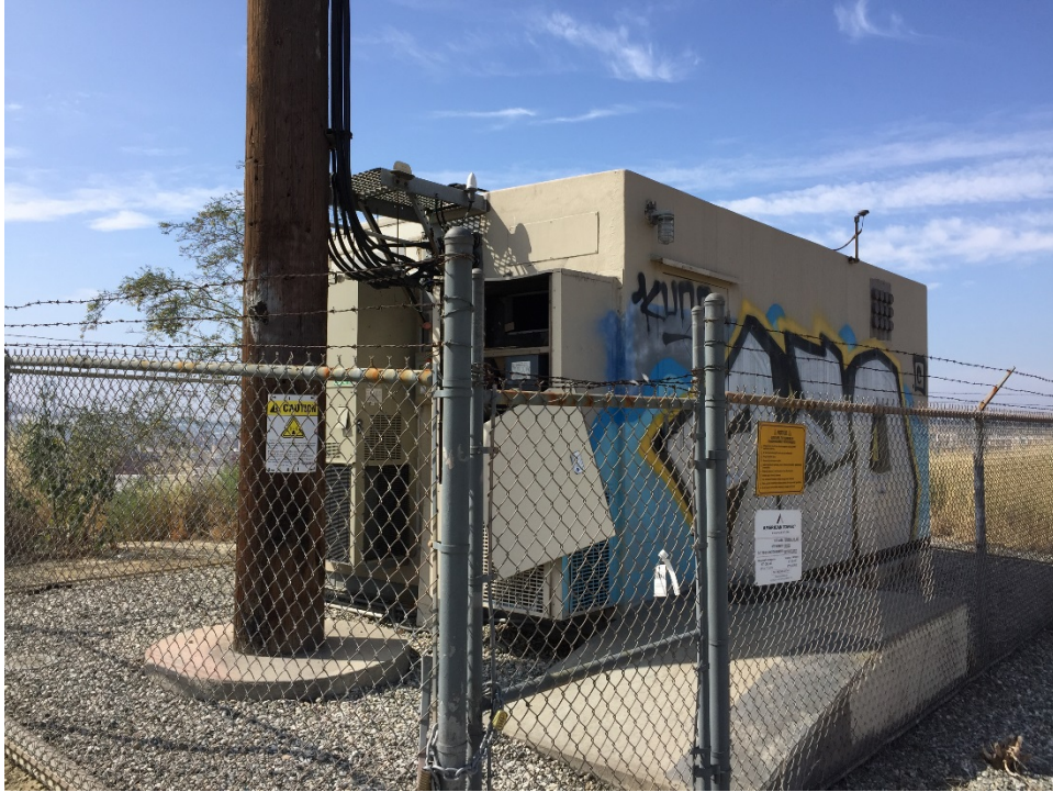
Photo 19 – The eastern cell tower and associated electrical building on the Property.
