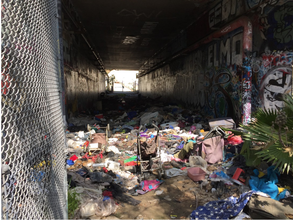
Photo 43 – Culvert beneath the freeway filled with trash and evidence of a homeless encampment.
