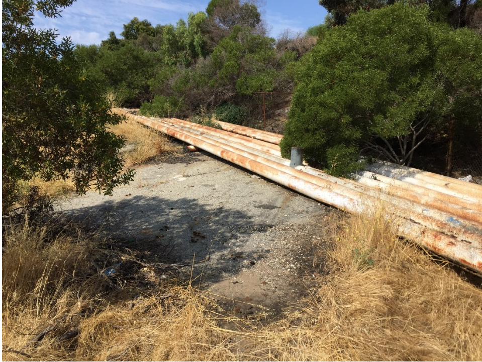
Photo 27 – A small asphalt-paved area and pipelines on the northwestern edge of the Property.
