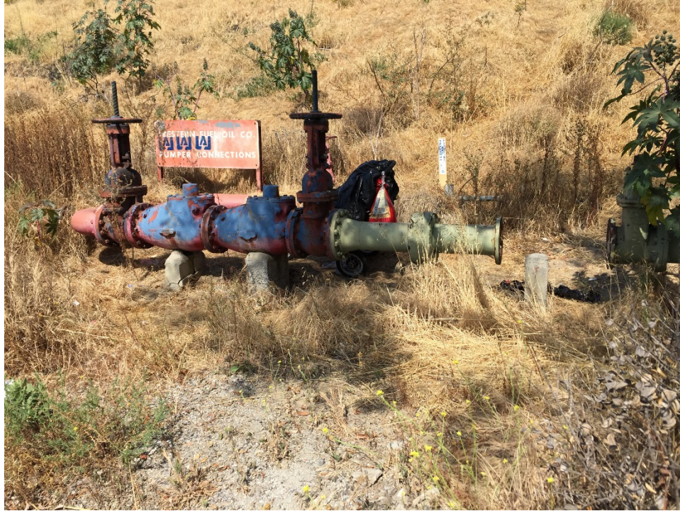
Photo 47 – Western Fuel Oil Company pumper connection equipment on the northern portion of the Property, along the edge of John S. Gibson Boulevard.
