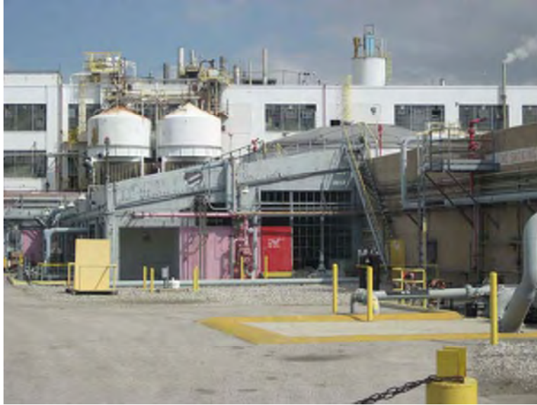
Photograph 6. View of the pump house, view to the north.
