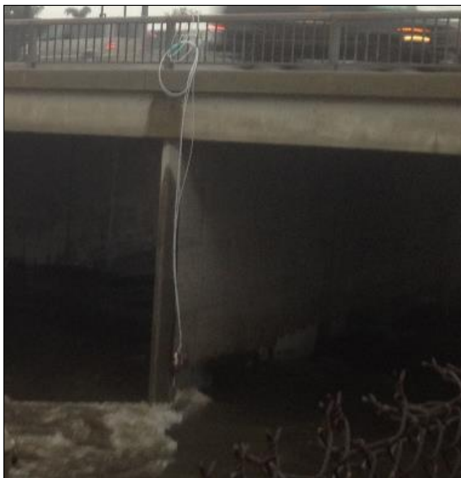
A battery of sample intakes was installed on the Artesia Blvd. Bridge.
