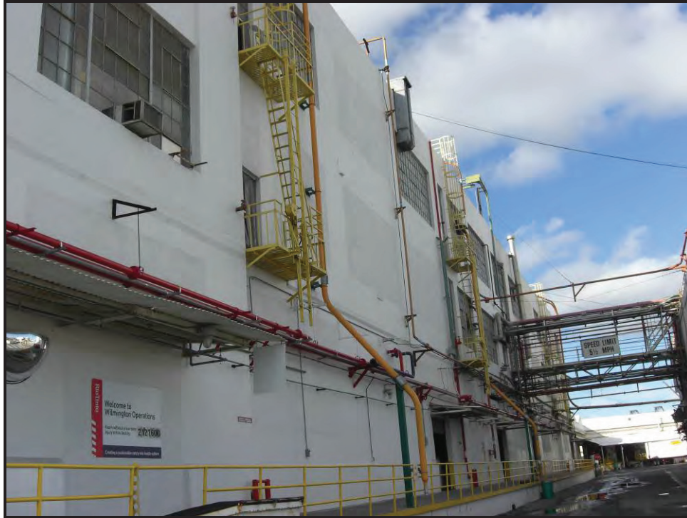
Detail of in-filled windows and non-historic equipment on north elevation of Refinery Building.
