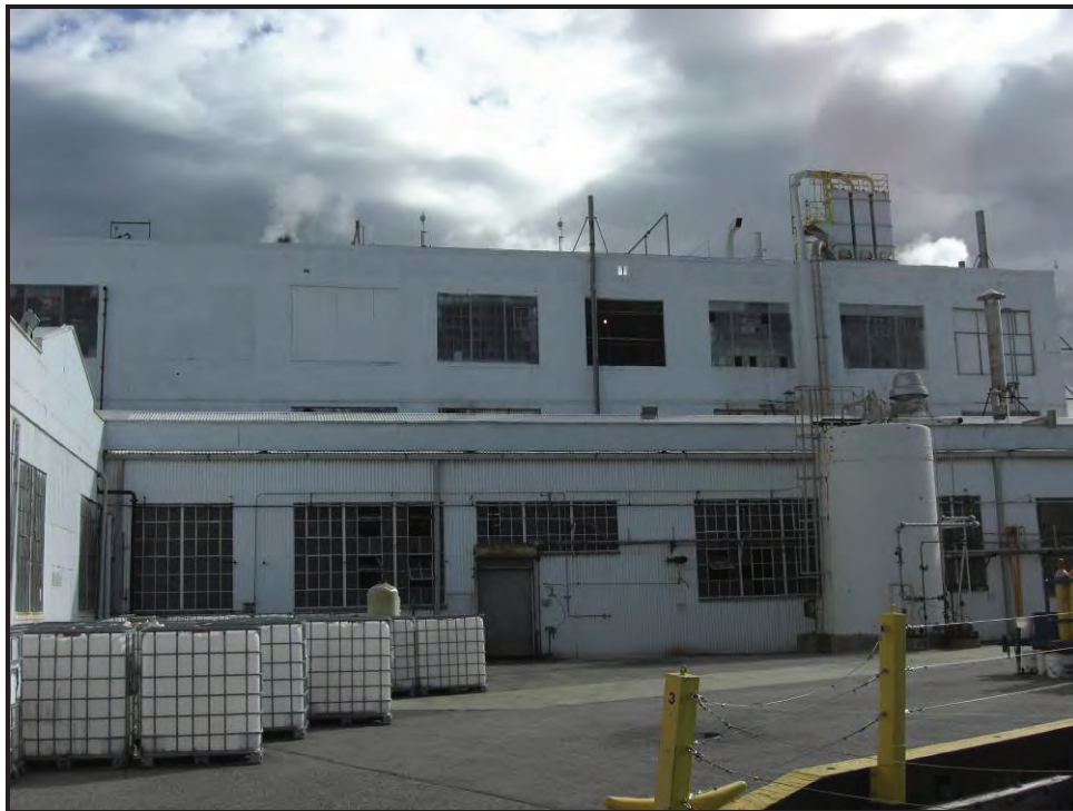
Detail of in-filled windows, non-historic equipment and addition on west elevation of Refinery Building.
