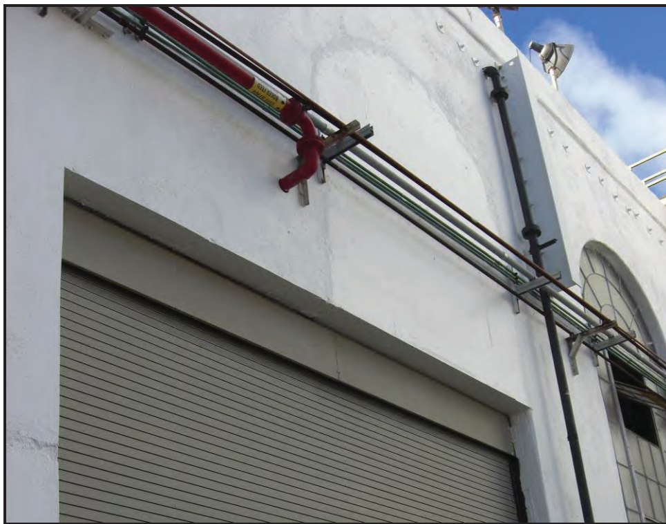
Detail of non-historic period metal roll-top door and window infill on north elevation of Power Plant.
