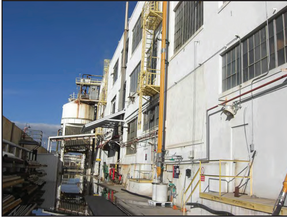
Detail of in-filled windows and non-historic equipment on south elevation of Refinery Building.
