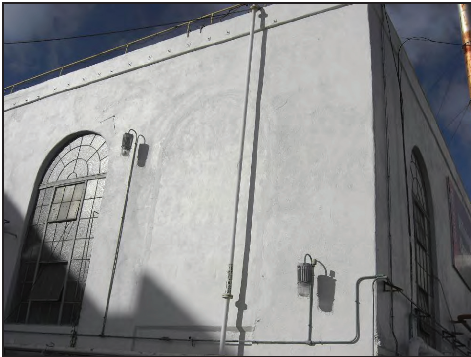
Detail of in-filled window and non-historic period utilities added to Power Plant.
