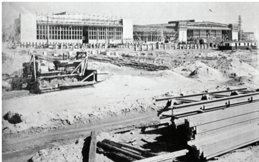
Figure 10. Building 5 under construction, April 1940. Courtesy of the National Archives Pacific Region, San Bruno
