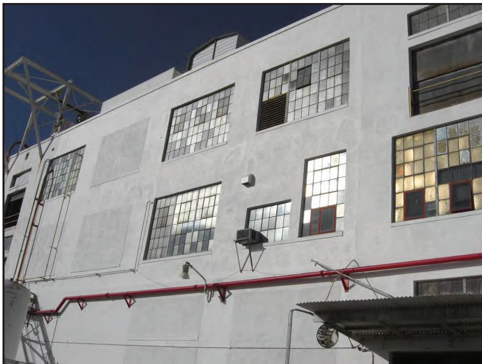
Detail of in-filled windows and non-historic equipment on east elevation of Refinery Building.
