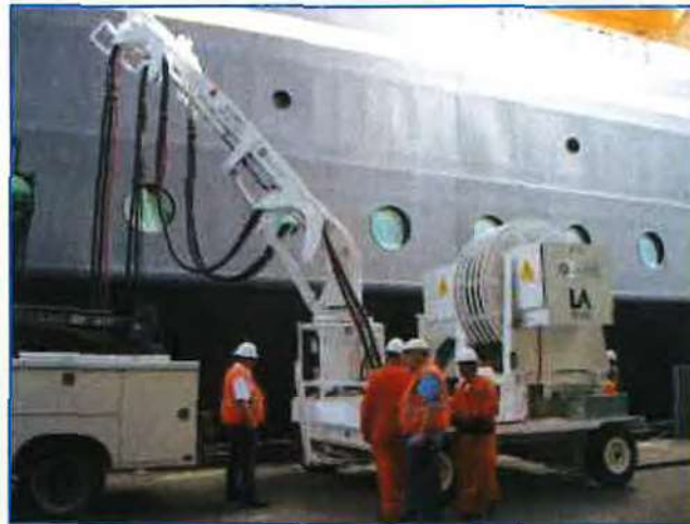
PowerMove - mini connected in Los Angeles (in use from 2009)
