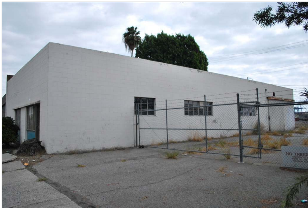
Figure 22. Rear (west) building of the Net Shed Storage Complex; view facing southwest, 2014.
