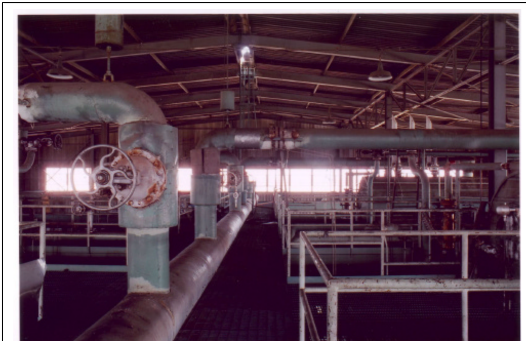
Canner's Steam Company Plant, View of Steam Pipes
