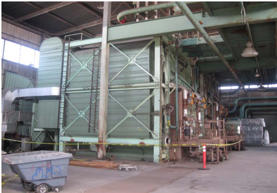
Photograph 6. Canner's Steam Company Plant, Interior, View of Boilers
