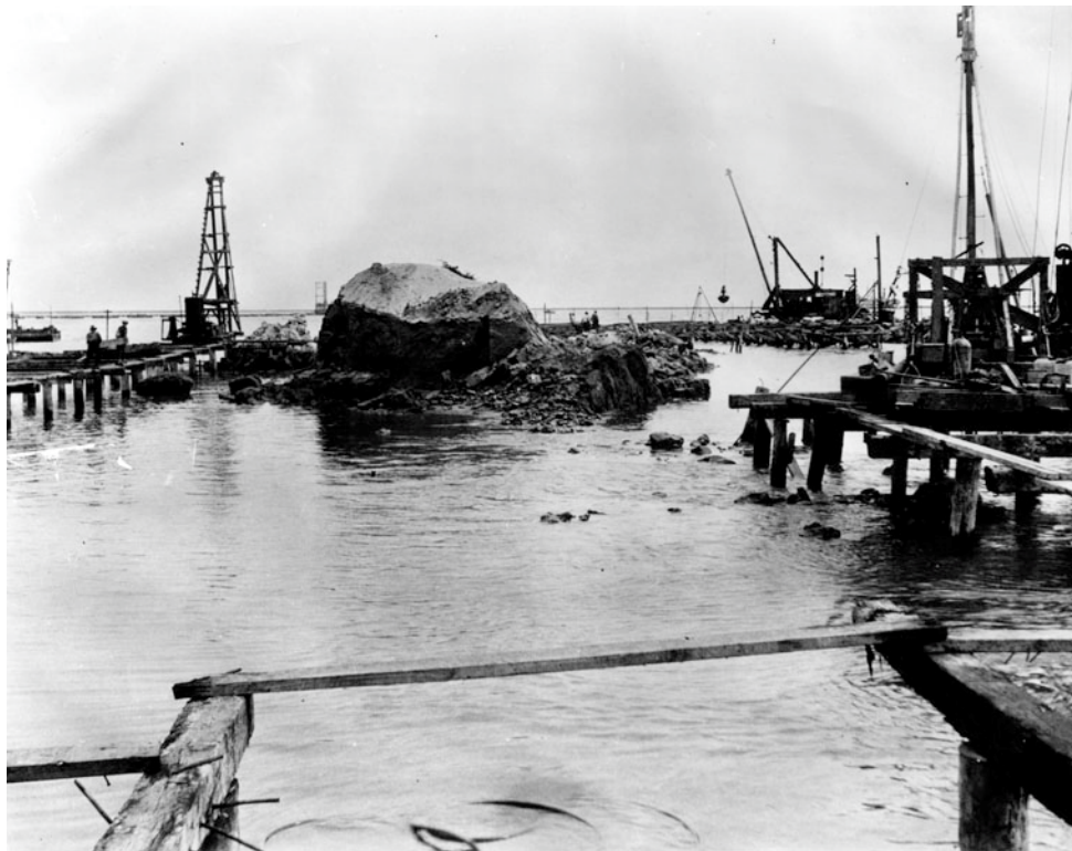
Figure 4. Demolition of Dead Man's Island, dredging and infilling to create Terminal Island ca. 1920 (Los Angeles Water and Power Associates Photo Archive).
