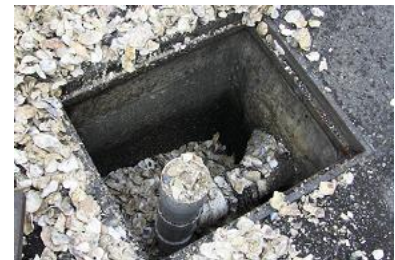
Figure 7. Oyster shells in a modified storm drain inlet at the Port of Seattle
