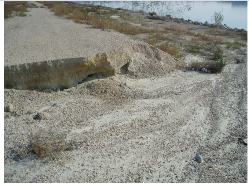
Berth 306, runoff channel (~5 ft deep) perpendicular to shore.
