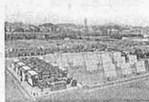
Integrated 1 MW solar photovoltaic and battery storage system (terminal functions as a green microgrid)
