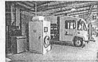
Standardized bi-directional charging systems
