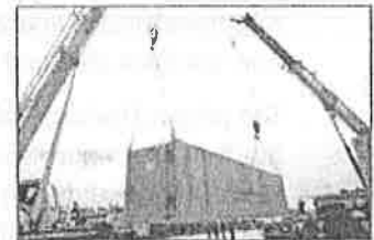
BYD BATTERY STORAGE SYSTEM
