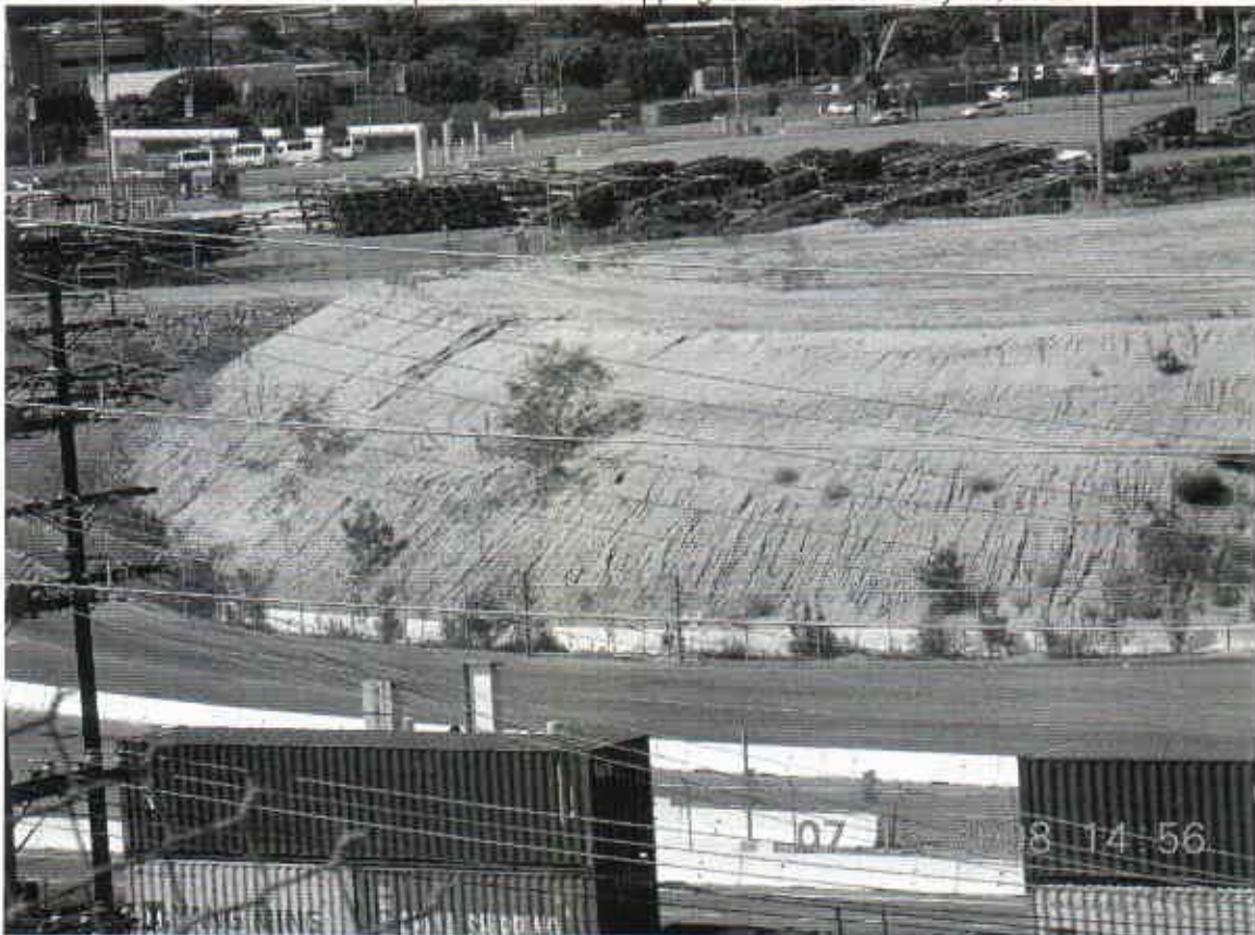
Water Erosion Impacts – China Shipping Landfill Site – July 13, 2008
