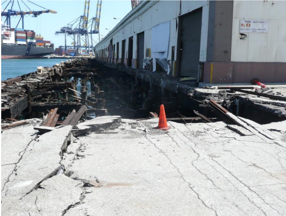
Figure 2-4c. Fire-Damaged East Façade of Building and Wood Wharf
