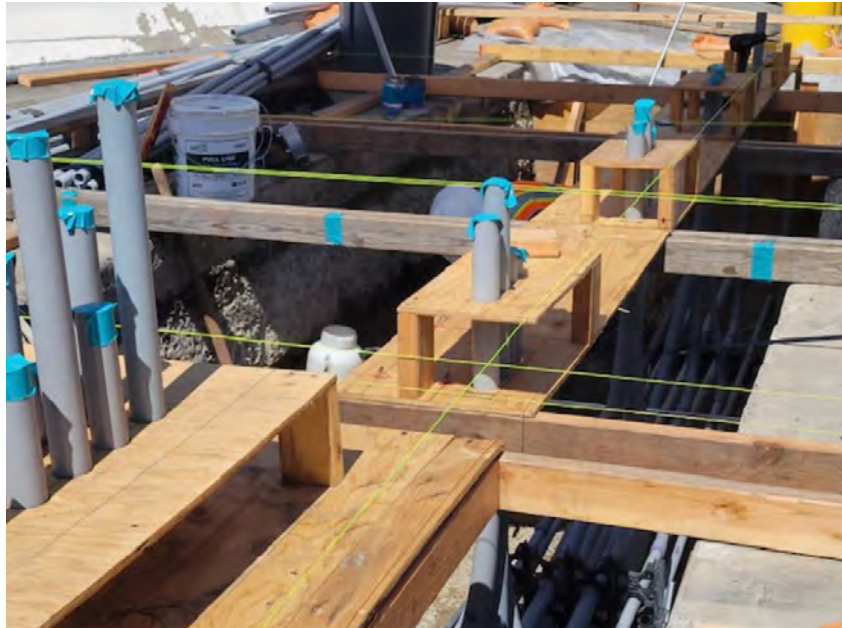
FIGURE 1: POLA Construction & Maintenance moved forward with site preparation to install the switchgear and BESS. Photos clockwise: battery cabinet conduits; west side of the substation; and inverter conduits.
