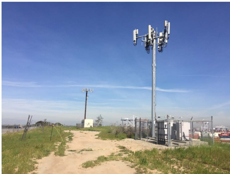
Cellular towers and associated electrical equipment located on the central portion of the site
