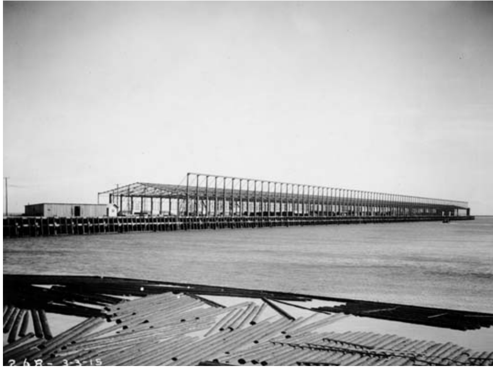
Photograph 6: Construction of Shed No. 1, 1915 (Los Angeles Board of Harbor Commissioner Annual Report -1914-1915)
