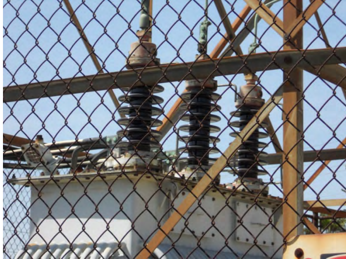
Plate 5. Electrical Insulators and Live Wires within Structure 1.
