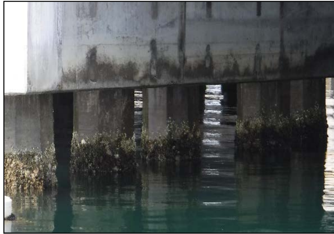
Figure 4.4-1. Pier Piling Biota, Rail Bridge (July 2018)
