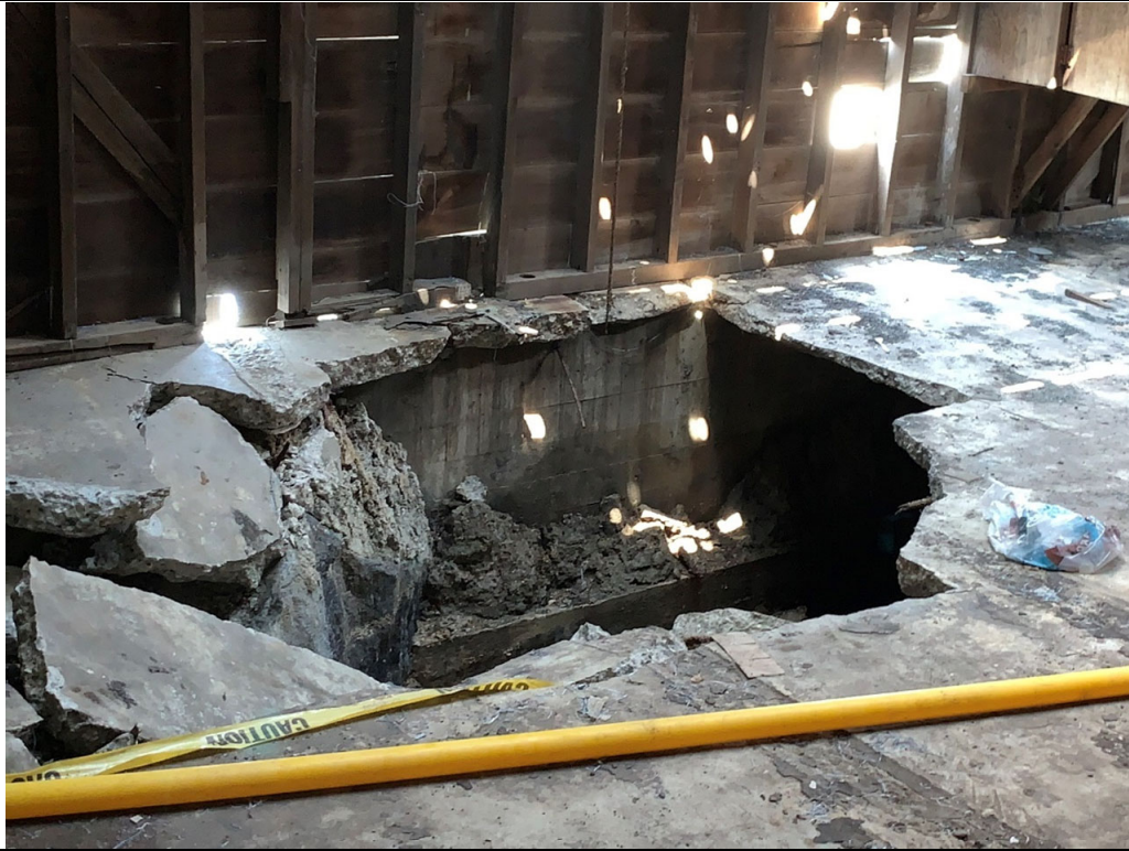
P-7 (Interior – Sinkhole, Seawall Visible)
