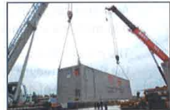
BYD BATTERY STORAGE SYSTEM
