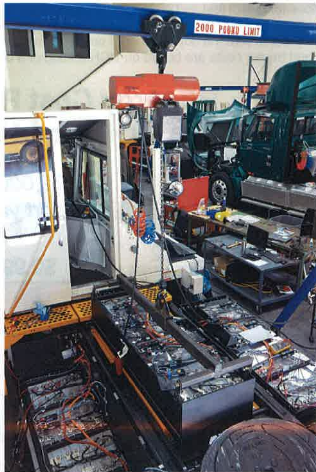
Figure 6. Battery enclosures installed on POLA-1.
