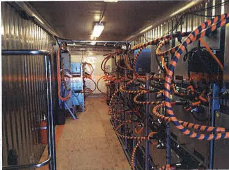
Figure 1. 1 MWh Grid-Saver™ system installed into a 45-foot trailer.
