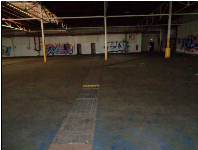
Figure 5-29. Star-Kist Plant No. 4, interior, warehouse/manufacturing area showing drains in floor, camera facing east.
