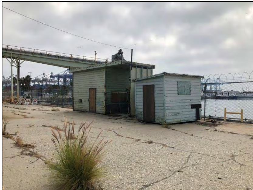
Figure 5-20. Star-Kist Plant No. 4, south elevation's ancillary/related buildings/structures, showing tuna import bridge in background, camera facing southeast.
