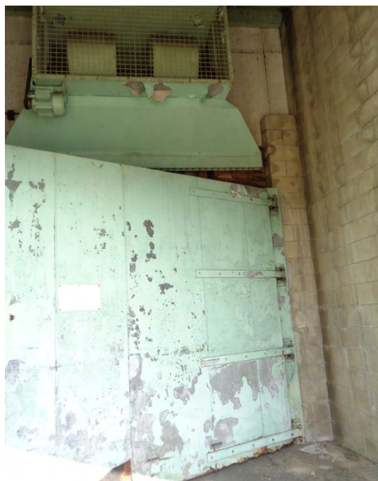
Figure 5-41. South elevation, Cold Storage portion of the facility, detail showing a cold storage door, camera facing northeast.
