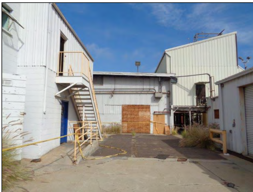
Figure 5-24. Star-Kist Plant No. 4, rear (east) elevation, detail of ancillary two buildings/structures (left, with staircase; right, with roll-up door) and warehouse/manufacturing building (center), camera facing north.
