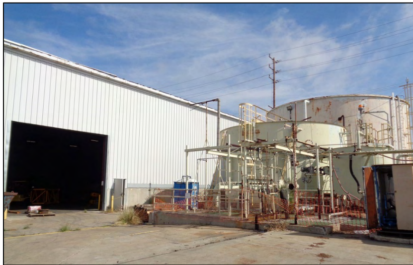
Photograph 4: South elevation, Cold Storage portion of the facility, camera facing northeast. ICF, 2018.
