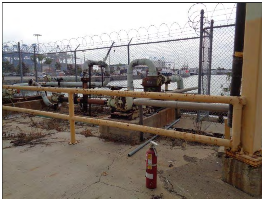
Figure 5-21. Star-Kist Plant No. 4, ancillary/related buildings/structures adjacent to south elevation, showing pipes, railings, fencing, and concrete pads, camera facing southeast.
