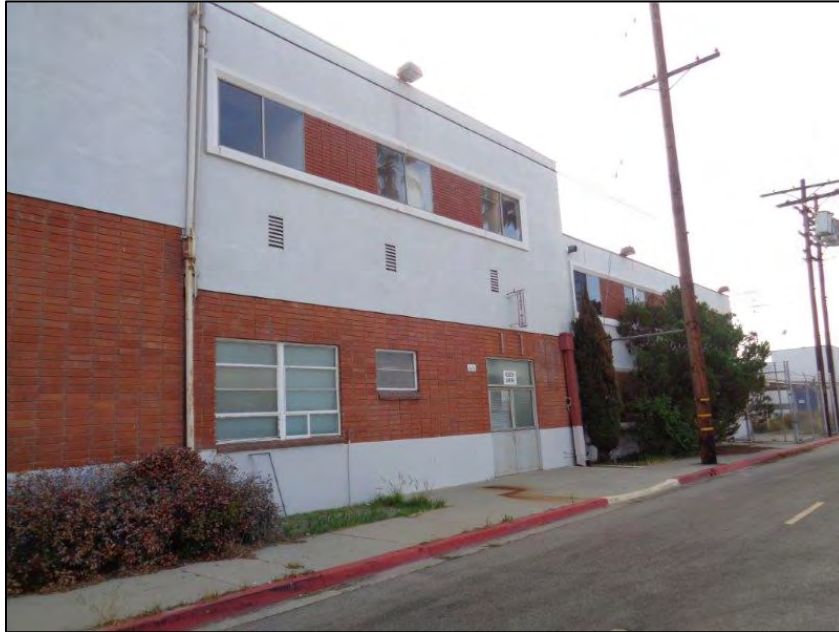
Figure 9: Star-Kist Plant No. 4, primary (west) elevation, detail of fourth volume from the north, camera facing southeast. ICF, 2018.
