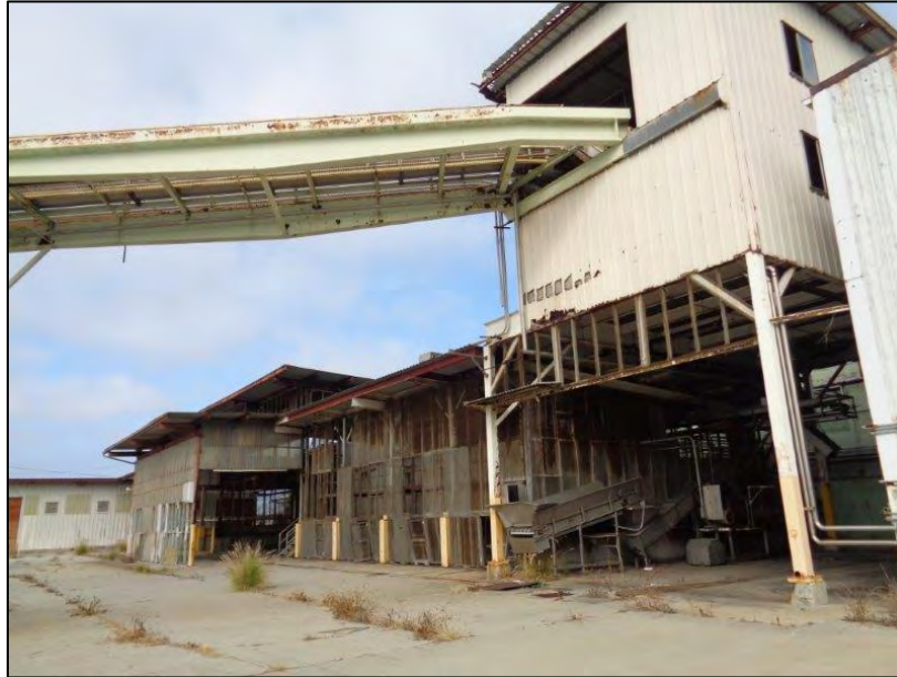
Figure 15: Star-Kist Plant No. 4, south elevation, southwest corner of Plant, showing tuna import bridge, camera facing northwest. ICF, 2018.
