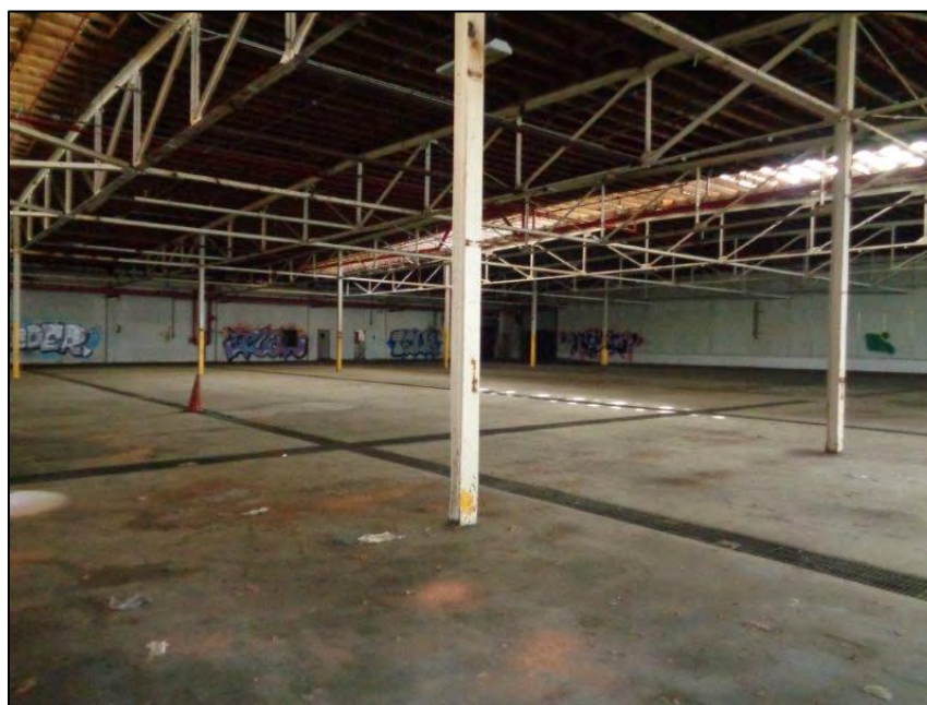
Figure 5-28. Star-Kist Plant No. 4, interior, warehouse/manufacturing area showing drains in floor, camera facing southeast.
