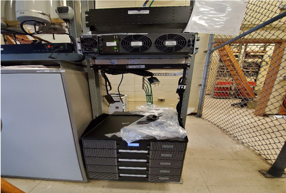
RACK SPACE 48 Units – Old Lease
