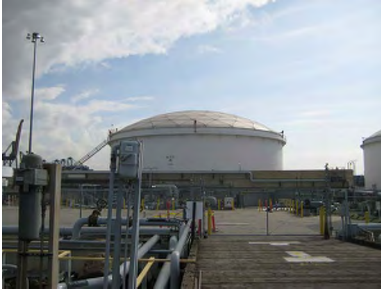
Photograph 4. View of storage tank M-10, view southeast.
