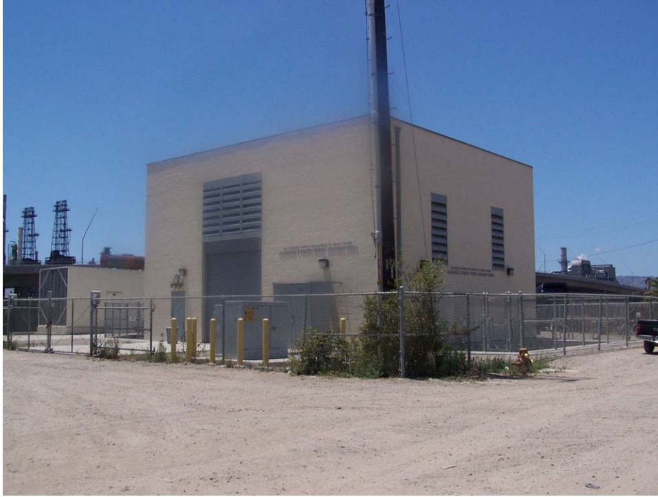
SW corner of East I Street and Wainwright Avenue. Southern California Edison substation.
