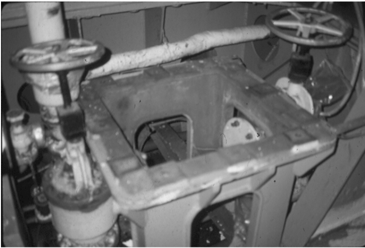
LUBE OIL PUMP FOUNDATION
