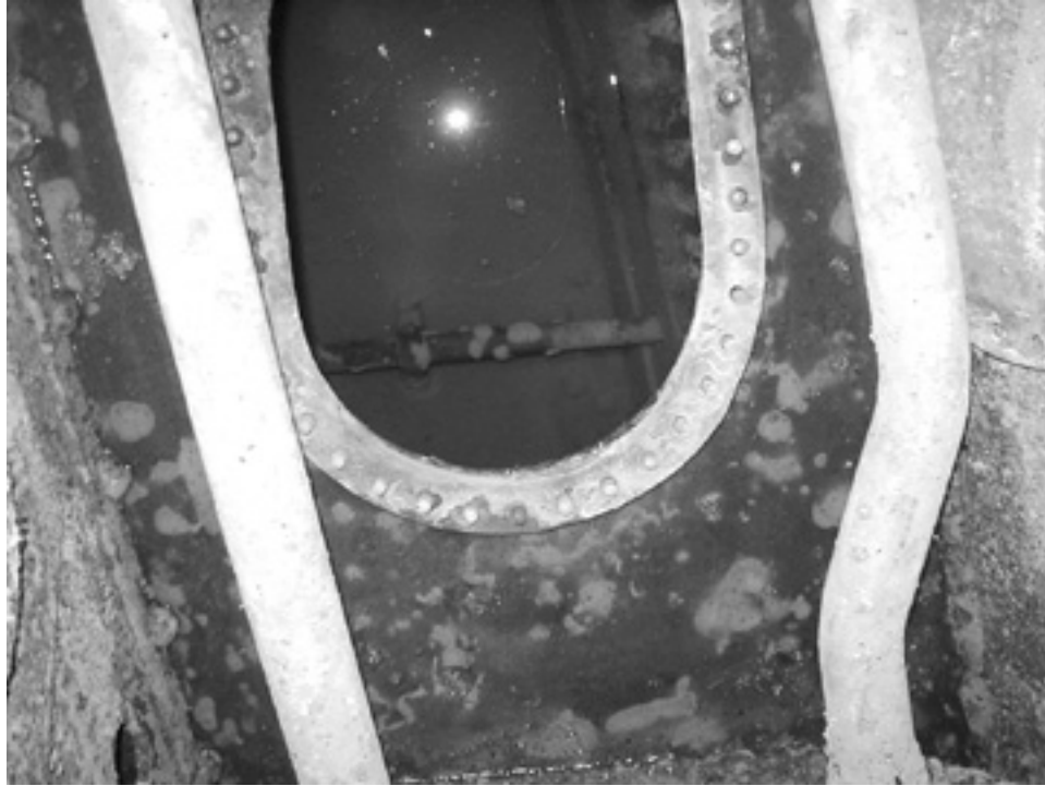
EXAMPLE OF DECK RUST AROUND MANHOLE
