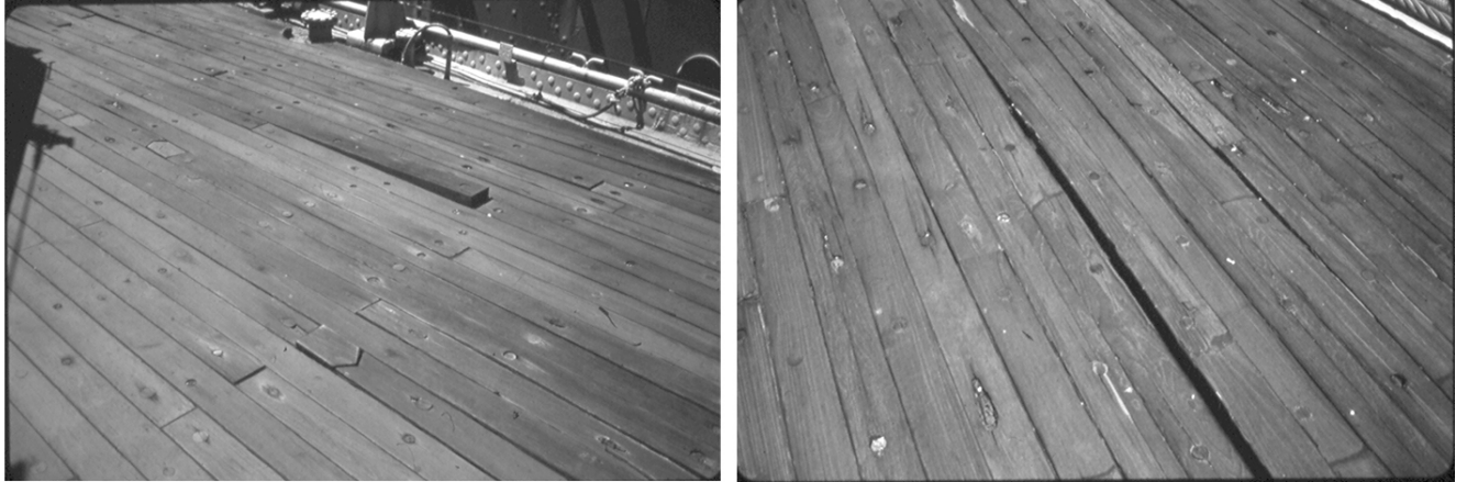
EXAMPLES OF WARPED AND ROTTED DOUGLAS FIR DECKING
