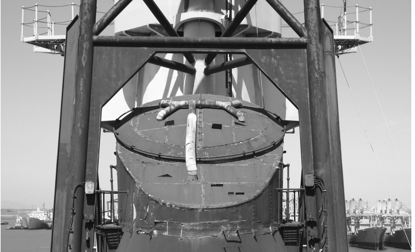
ROTTED D/H PIPING ON FWD STACK CAP.
