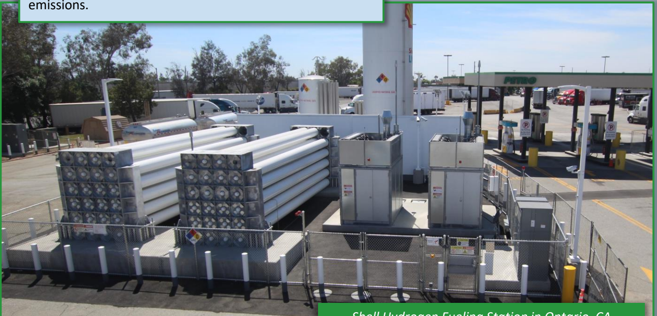
Shell Hydrogen Fueling Station in Ontario, CA
