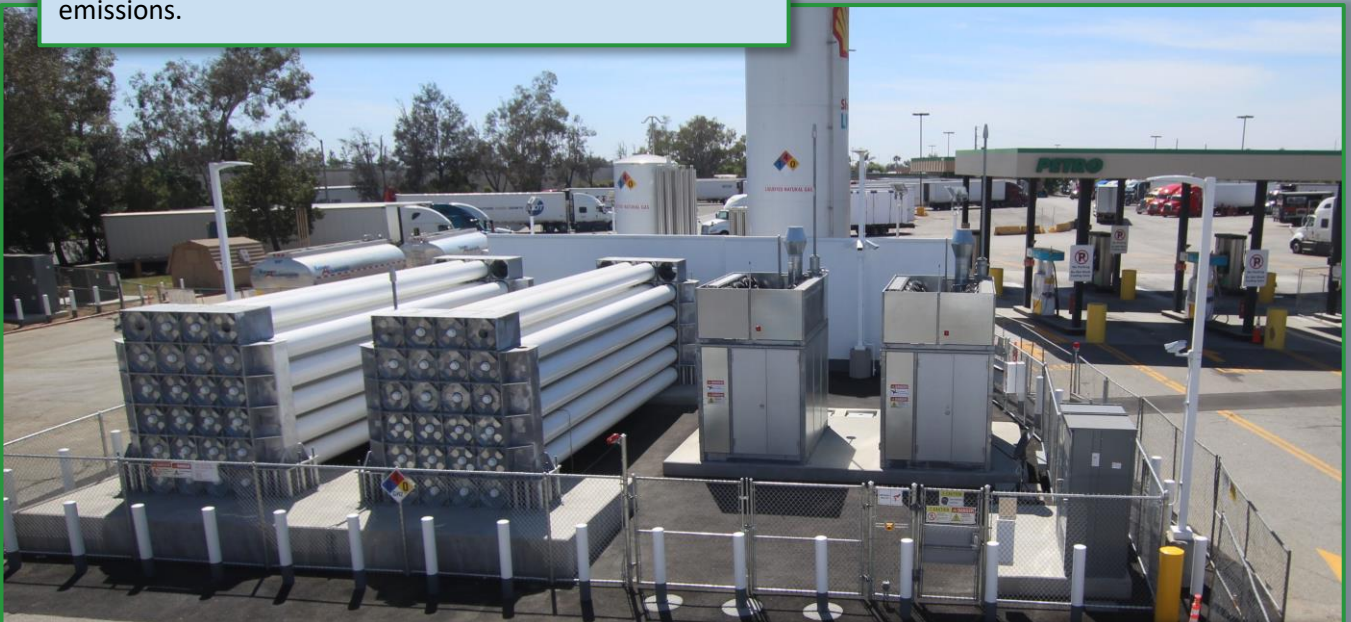
Shell Hydrogen Fueling Station in Ontario, CA
