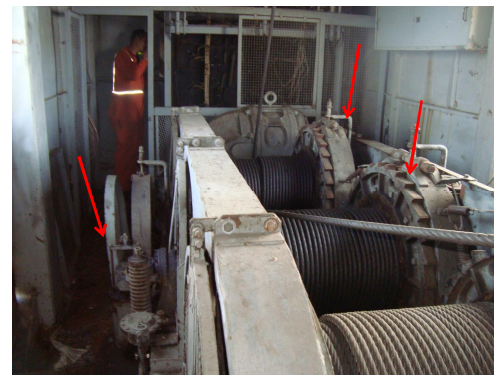
Main Hoist and Boom Hoist rope drums
