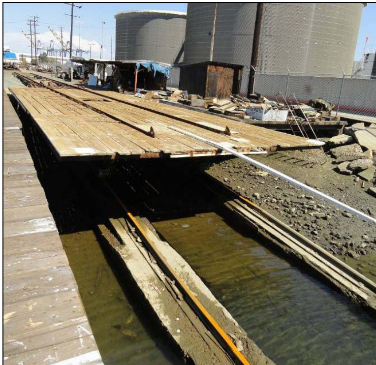
Figure 33 Marine ways, loading deck, winch shed, and shed roof storage building, looking east (Applied EarthWorks, August 29, 2012).
