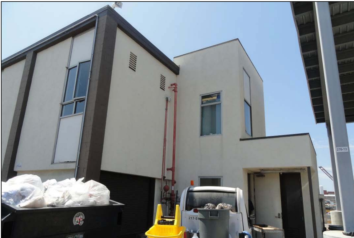
P5. Description of Photo: View looking north at the east facade addition on the Service Building.
