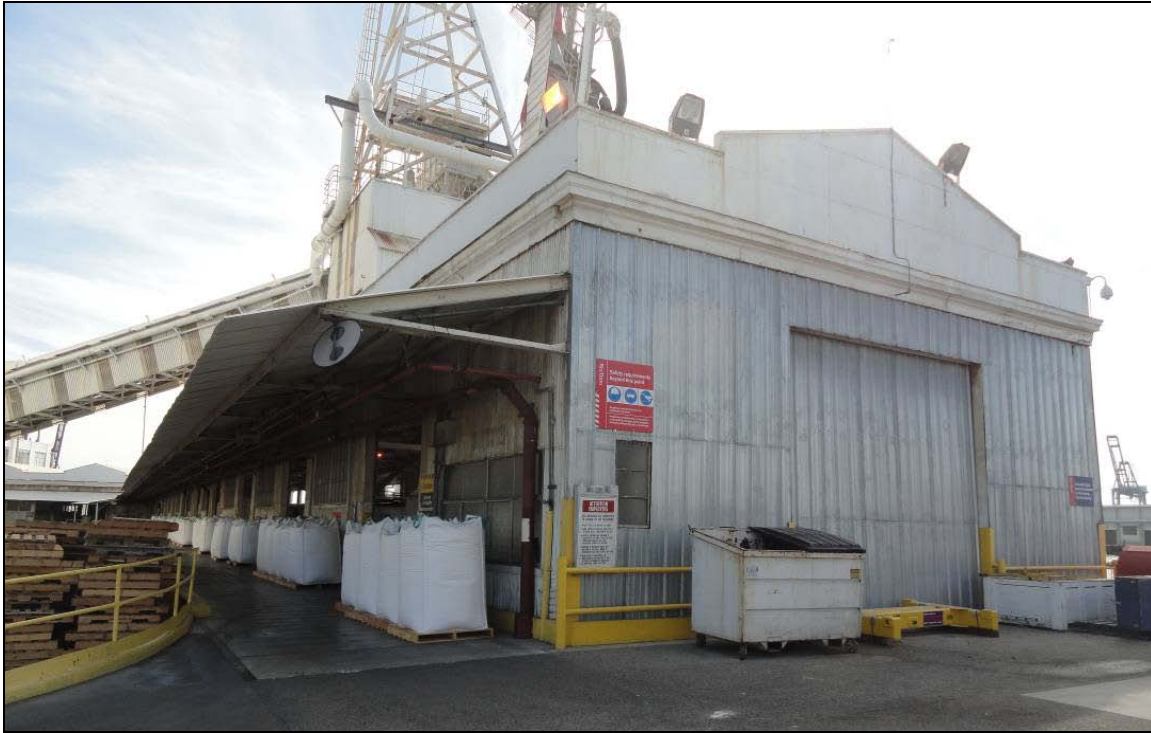
P5. Description of Photo: View looking south at the north and east façades of the warehouse.
