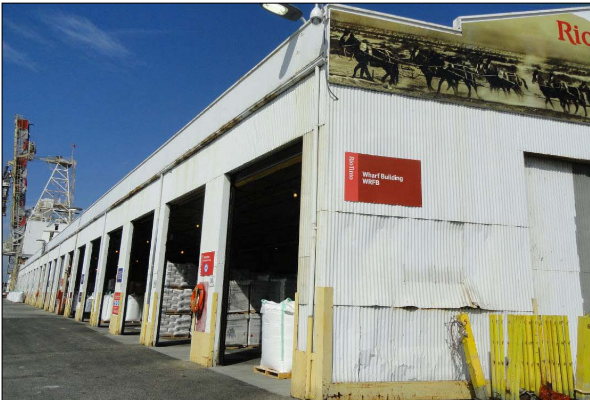
P5. Description of Photo: View looking north at the south and west façades of the warehouse.
