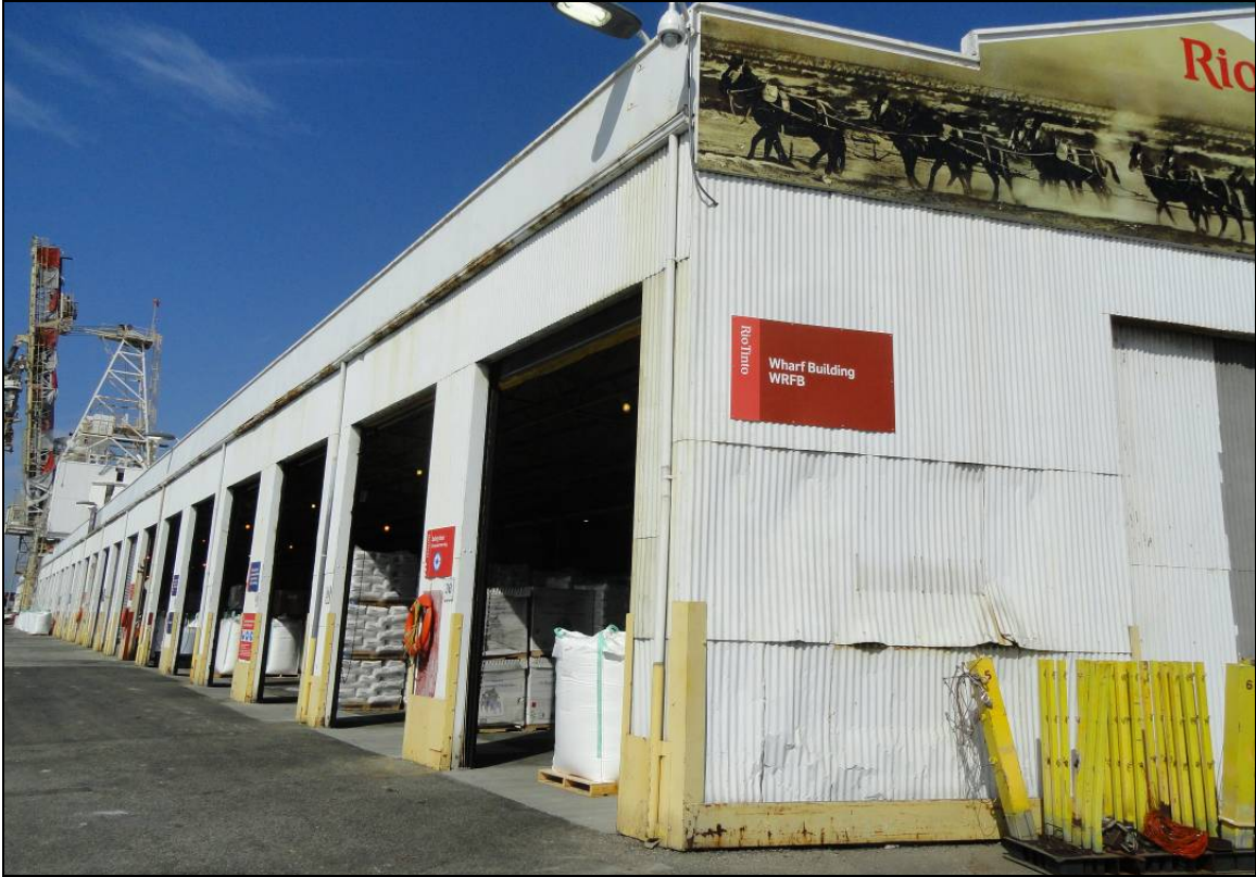
Figure 19 South and west facades of the warehouse, looking north (Applied EarthWorks, October 5, 2012).
