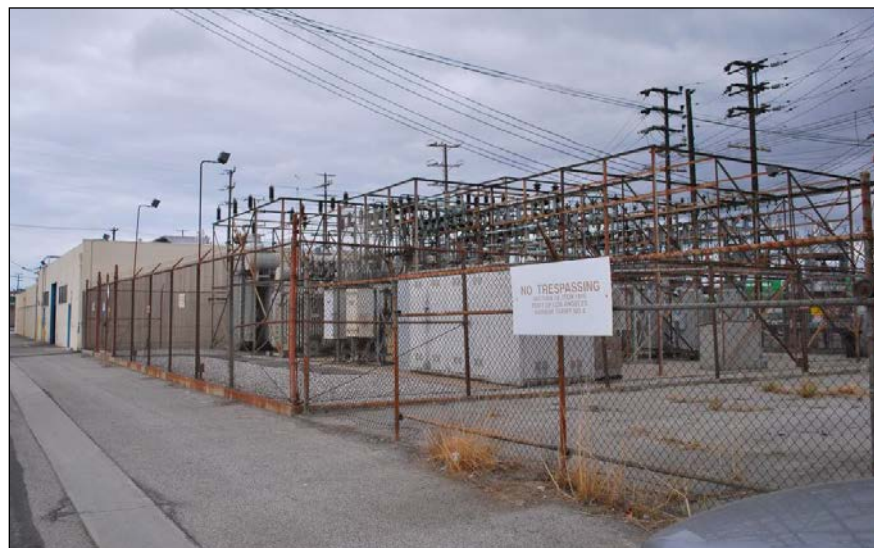
30 Photograph 3.4-9: Overview of Distribution Station 121; view facing 31 northwest, 2014
