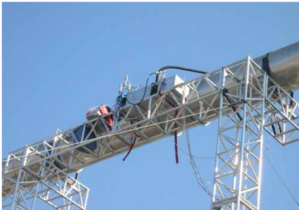
Figure 24. RAVEM Setup at the Inlet to the Emissions Treatment Subsystem
