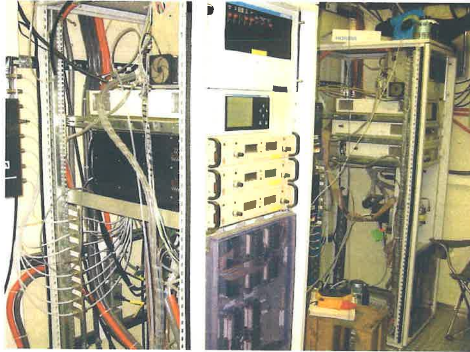
Figure 11. Continuous Emission Monitoring System
