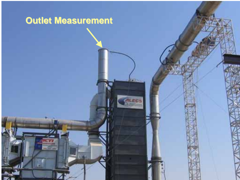
Figure 21. Exhaust Stack of the Emissions Treatment Subsystem
