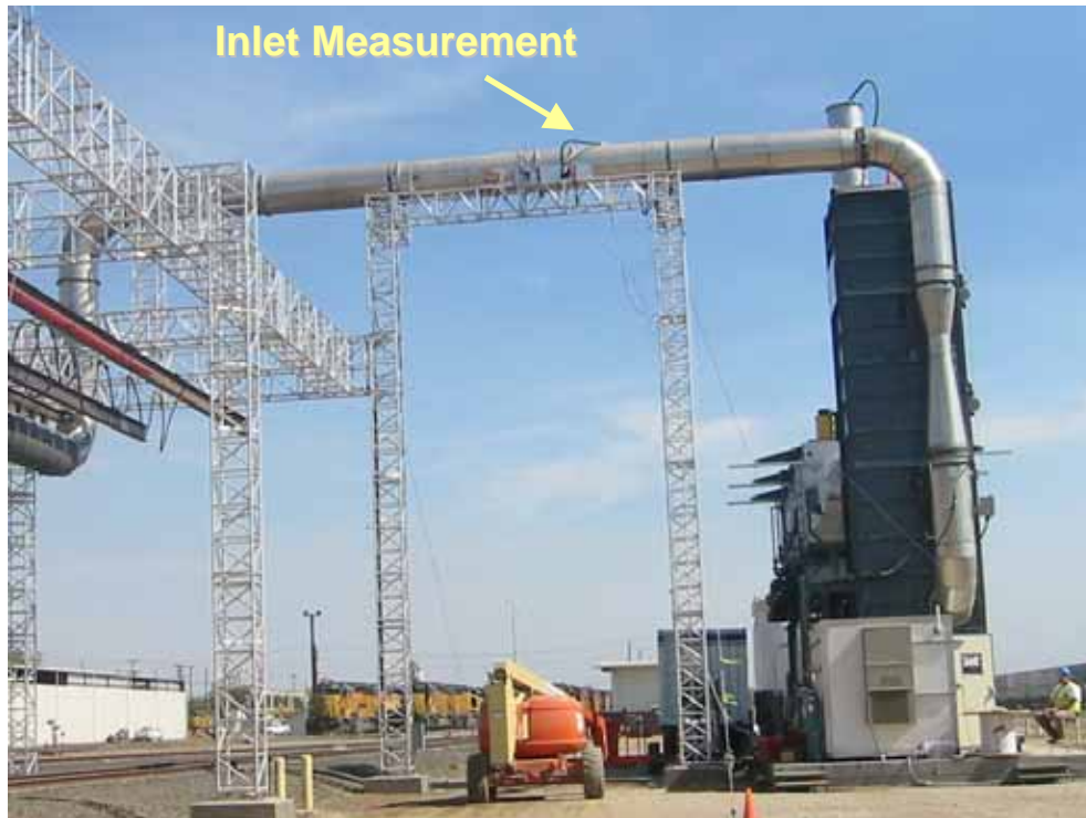
Figure 20. Ducting between the ECS and the ETS
