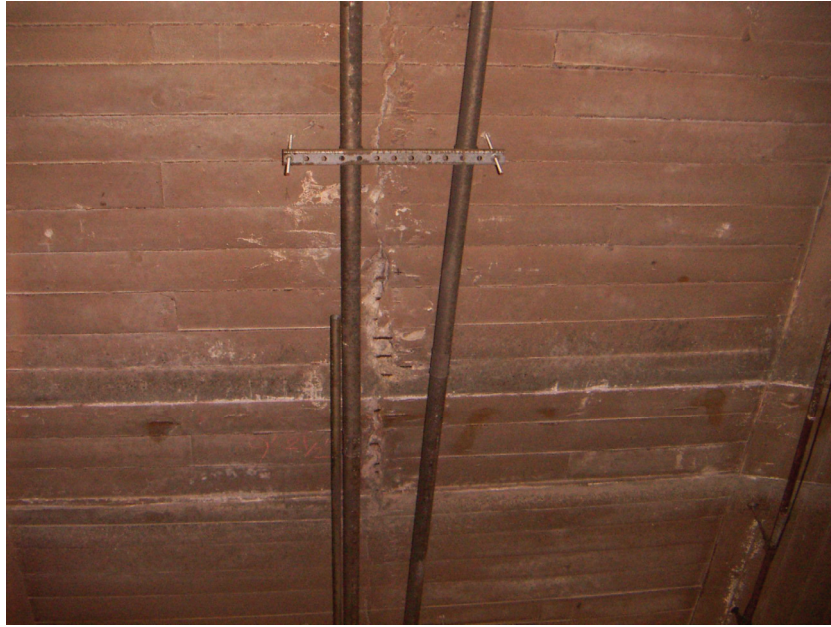
Figure 2 – Floor Crack at Ceiling of First Floor
