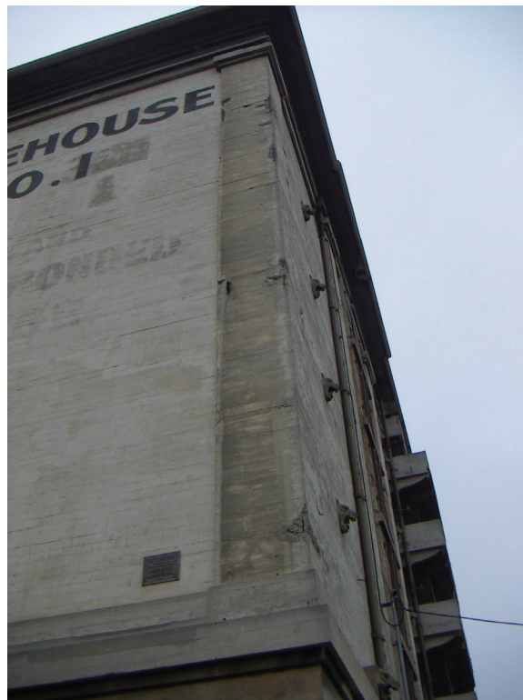
Figure 9 – Northwest Corner Deterioration & Historical Plaque
