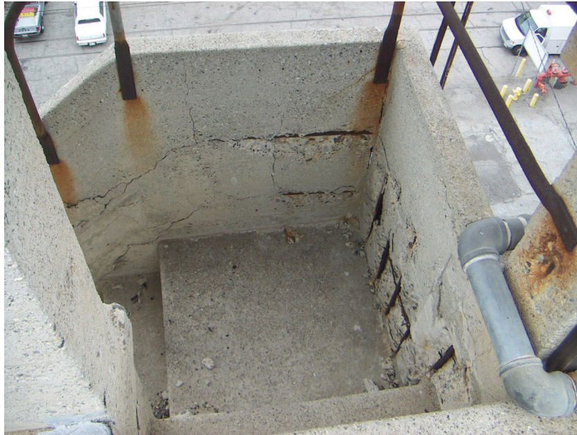
Figure 6 – Exterior Stair Deterioration
