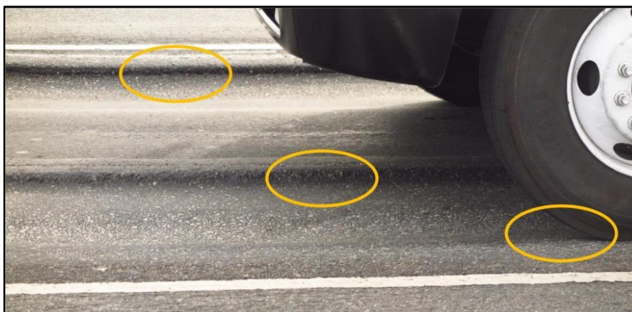
Figure 33 Lane grooves on Alameda Street at intersection
