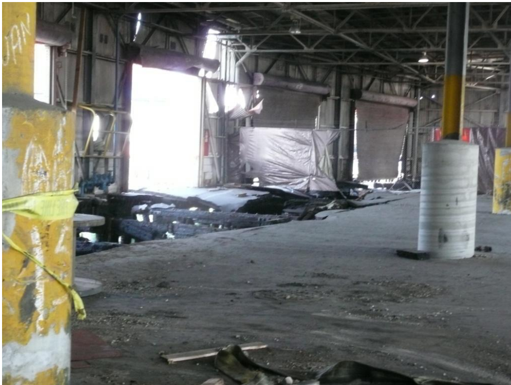
Figure 2-4d. Collapsing Floor and Fire-Damaged Metal Roll-up Doors
