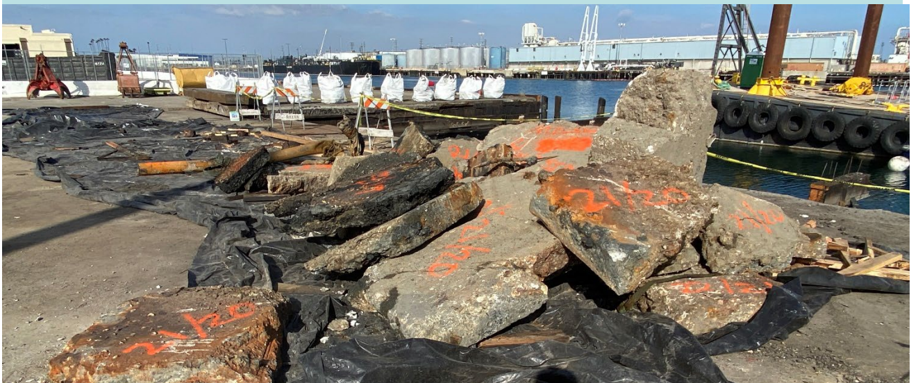
2/14/24 - Miscellaneous Debris Removal at Berth 178, Bents 21-23. Misc. 6" pipe, Concrete and Asphalt sizes vary from 1.5'x1.5'x6" to 3'x10'x8"
