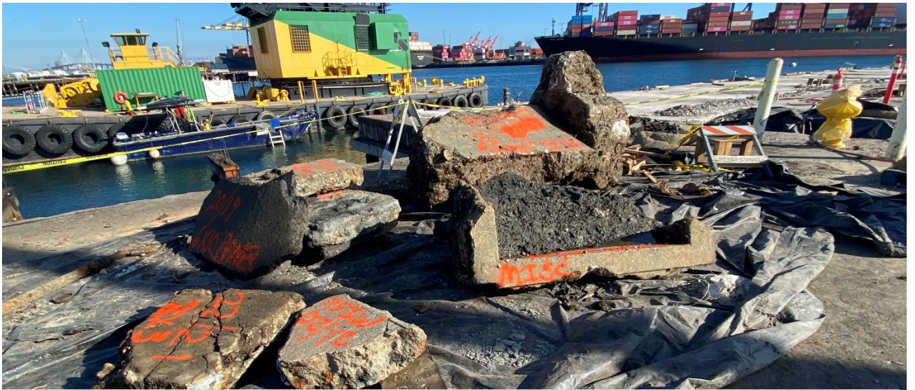
2/13/24 - Miscellaneous Concrete and Asphalt Debris Removal at Berth 178, Bents 20-23. Sizes vary from 1.5'x2'x6" to 8'x3'x3'
