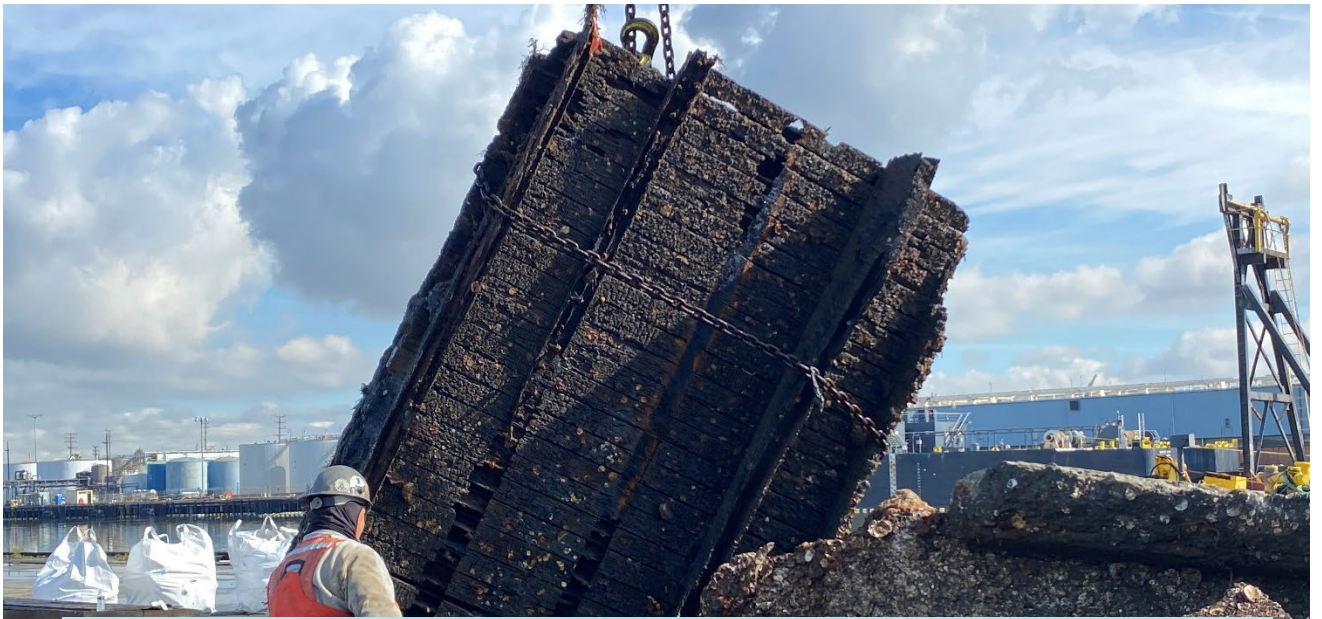
2/21/24 - Fallen Timber/Asphalt Deck Panel at Berth 178, Bents 17-18. Size is 12'x12'x9"
