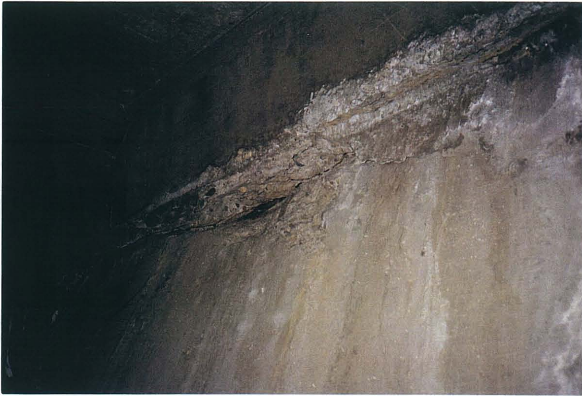
PHOTO 14-3. Crack and small gap between top of retaining structure (gravity wall) and bottom of rear marginal beam, indicating that retaining structure is setting. (Note that the structure was constructed with a cold joint between the two.)
