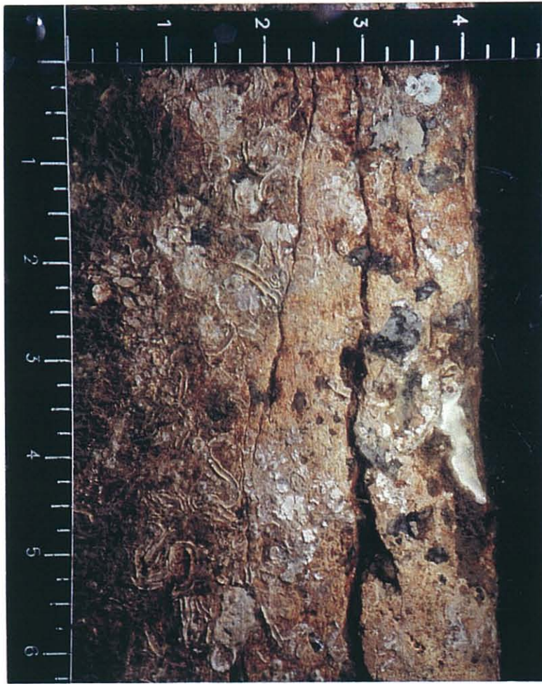
PHOTO 11-20. Underwater Corrosion cracks at corner of concrete pile.
