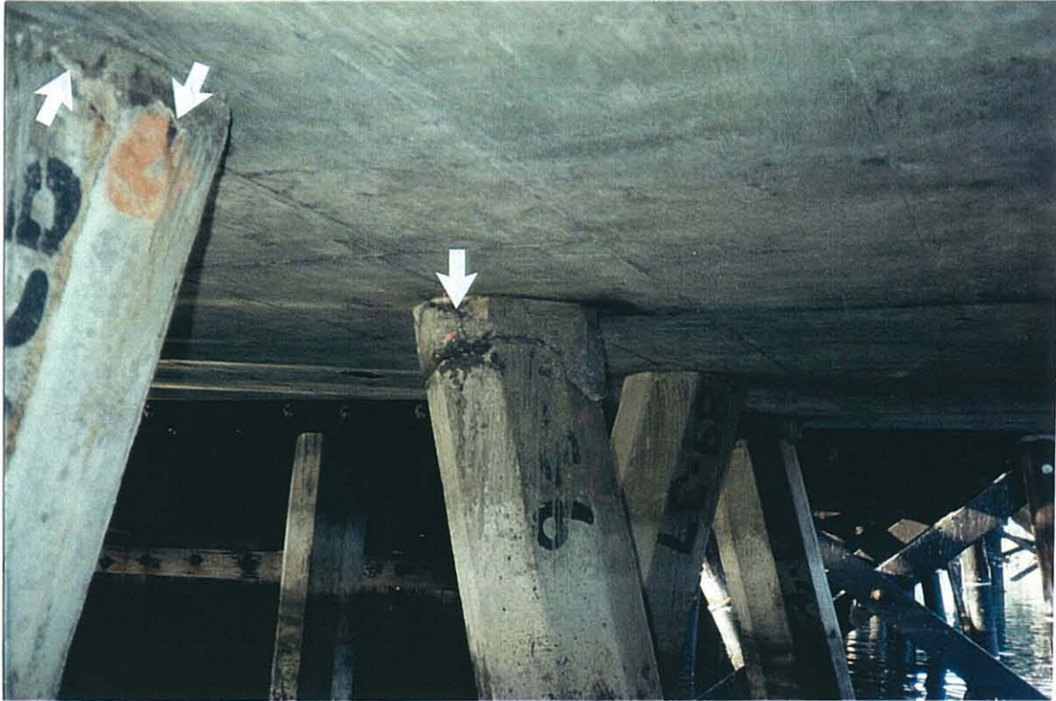
PHOTO 11-8. Overstressing cracks at top of batter pile, immediately below connection to deck.
