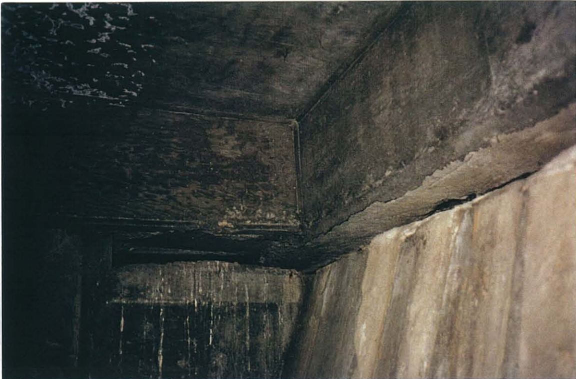
PHOTO 14-1. Gap between top of retaining structure (gravity wall) and bottom of rear marginal beam (right side of photo). Also note gap between top of diaphragm and bottom of pile cap (left side of photo).
