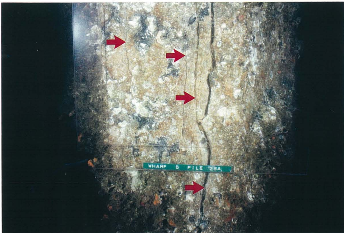
PHOTO 11-17. Several vertical underwater cracks on side of octagonal prestressed pile at elevation – 15 ft (courtesy of U.S. Navy/Blaylock Engineering Group).
