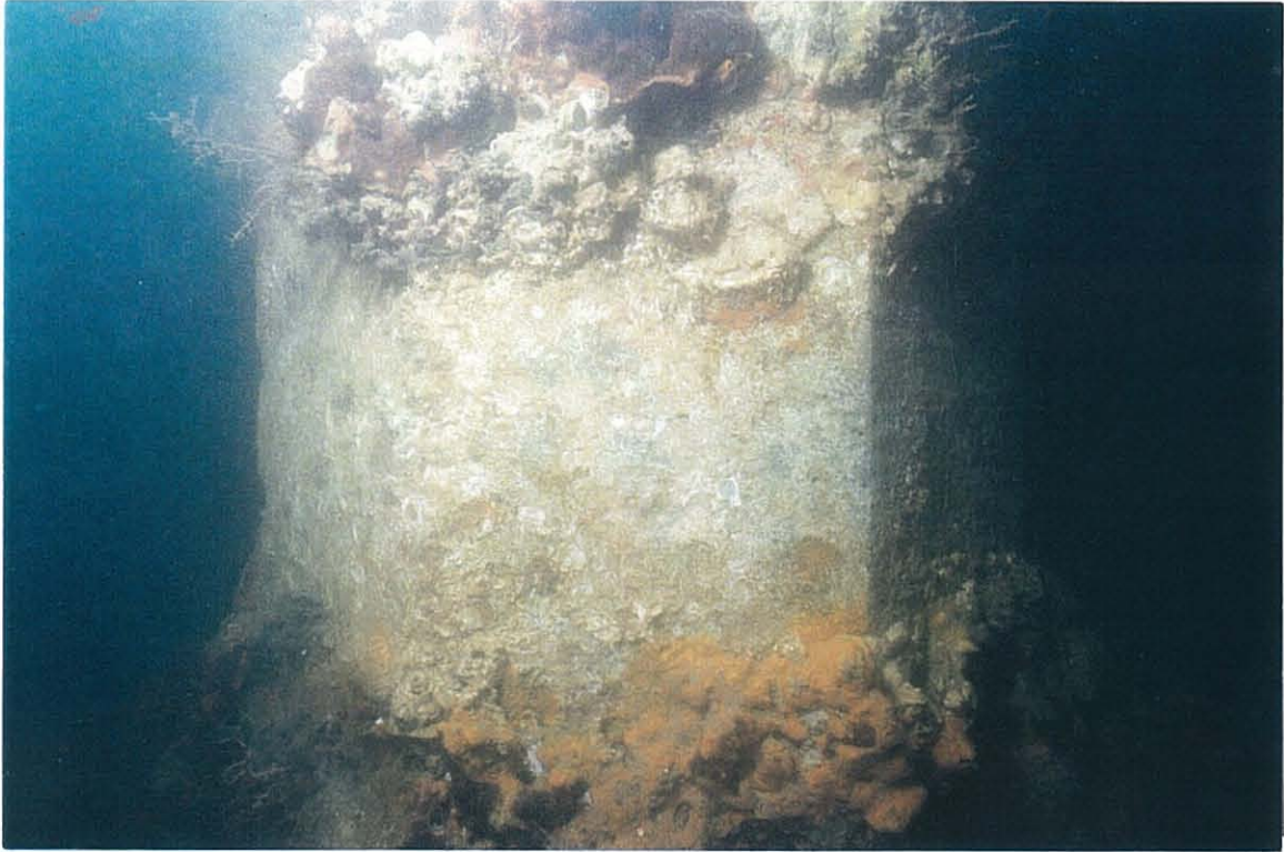
PHOTO 11-18. Approximately 12-in. high band, cleaned of marine growth for underwater Level II Inspection of prestressed pile.
