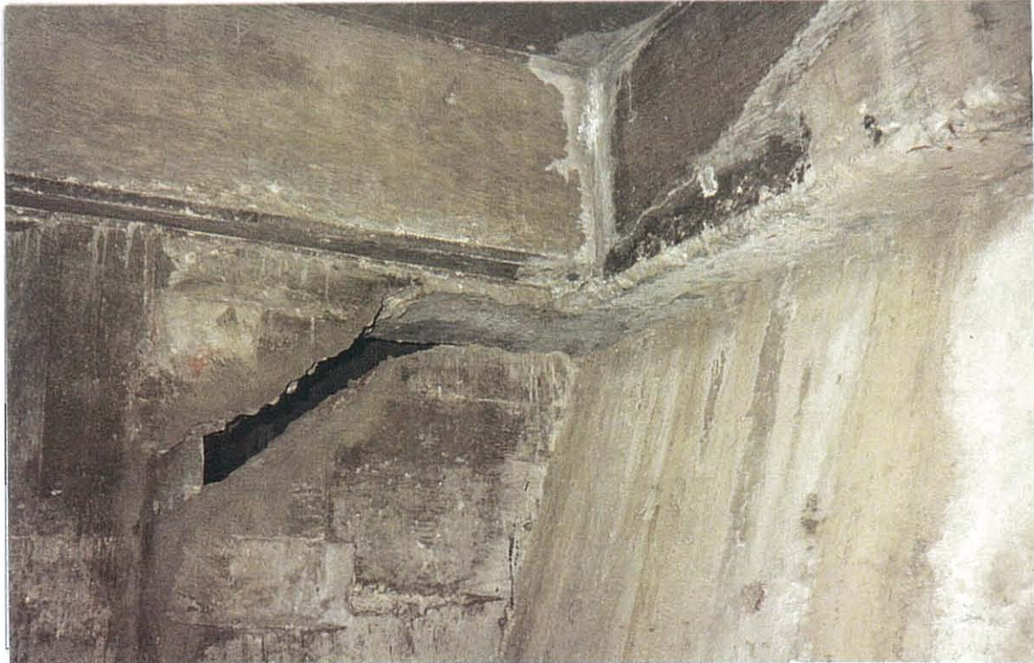
PHOTO 14-2. Gap between top of retaining structure (gravity wall) and bottom of rear marginal beam (right side of photo). Also note gap between top of diaphragm and bottom of pile cap, and a diagonal crack which has opened up into a gap in the diaphragm adjacent to pile (left side of photo).
