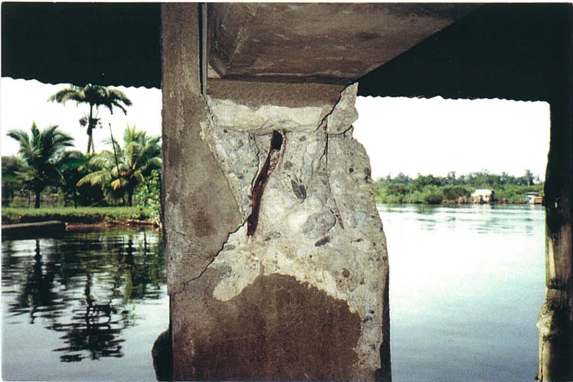
PHOTO 11-4. Breakage of concrete pile immediately below connection with cap.
