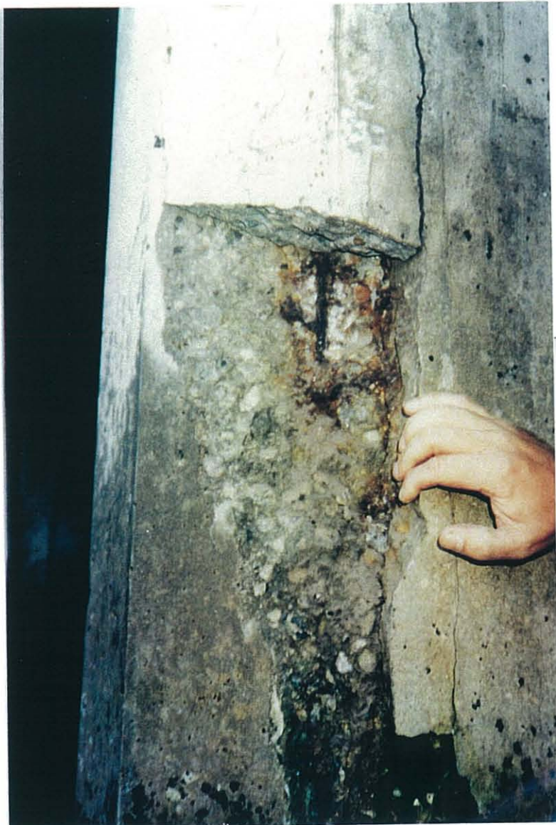
PHOTO 11-12 (left). Close up of corrosion crack shown in Photo 11-11 after removal of concrete cover. The prestressing strand which generated this crack is completely corroded.
