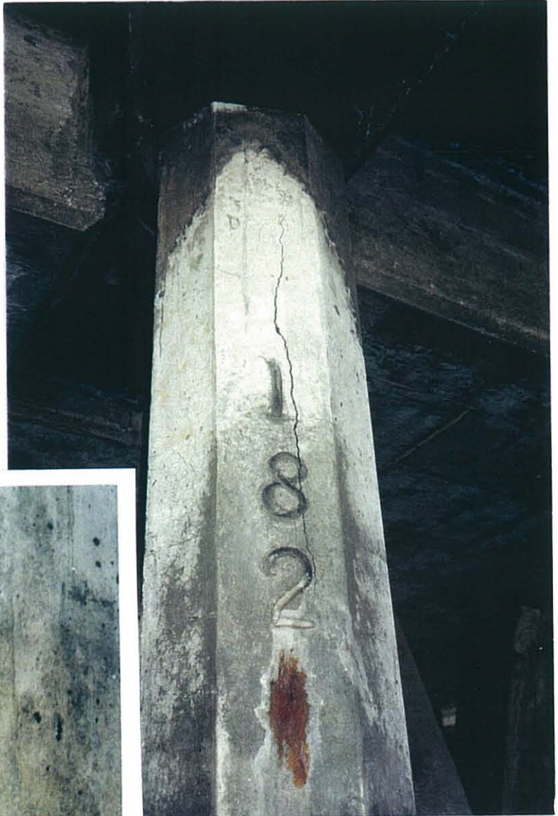
PHOTO 11-11 (right). Corrosion crack on prestressed pile.
