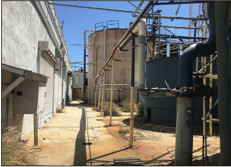
Figure 2: Cannery Block, pipes, tanks, and infrastructure elements, located at the northwest portion of block between a fence at Ways Street and a warehouse (shown on left), camera facing south. ICF, 2019.
