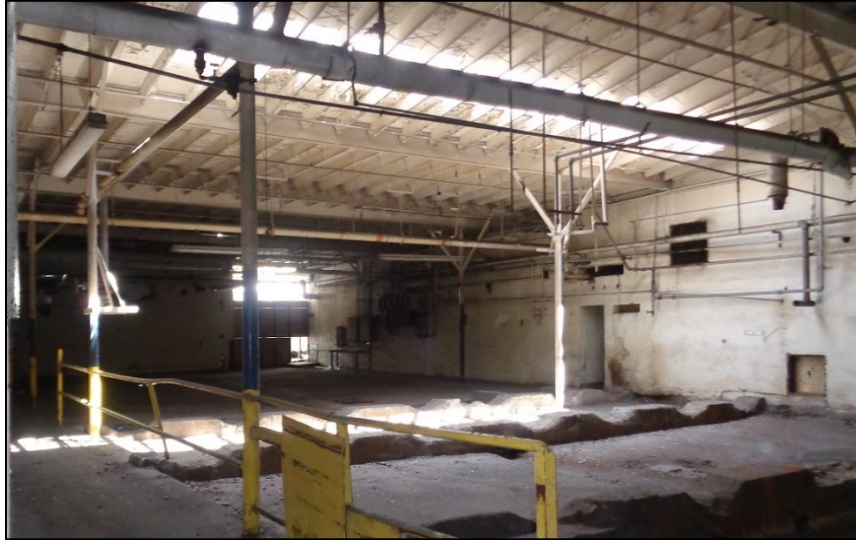
Figure 27: Cannery Block, 1953 warehouse interior, centered between Cannery Street and Sardine Street, just east of Ways Street, camera facing southwest. ICF, 2019.
