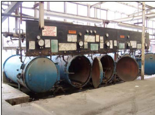
Figure 38: Cannery Block, retorts and associated mechanical infrastructure/operation board. ICF, 2006.
