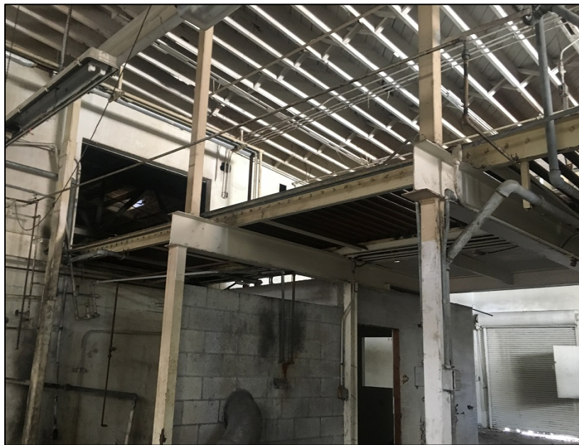
Figure 26: Cannery Block, 1951 warehouse interior, centered between Cannery Street and Sardine Street, just east of Ways Street, camera facing southwest. ICF, 2019.
