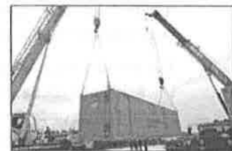
BYD BATTERY STORAGE SYSTEM
