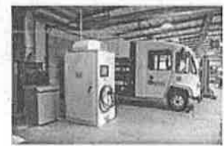
Standardized bi-directional charging systems
